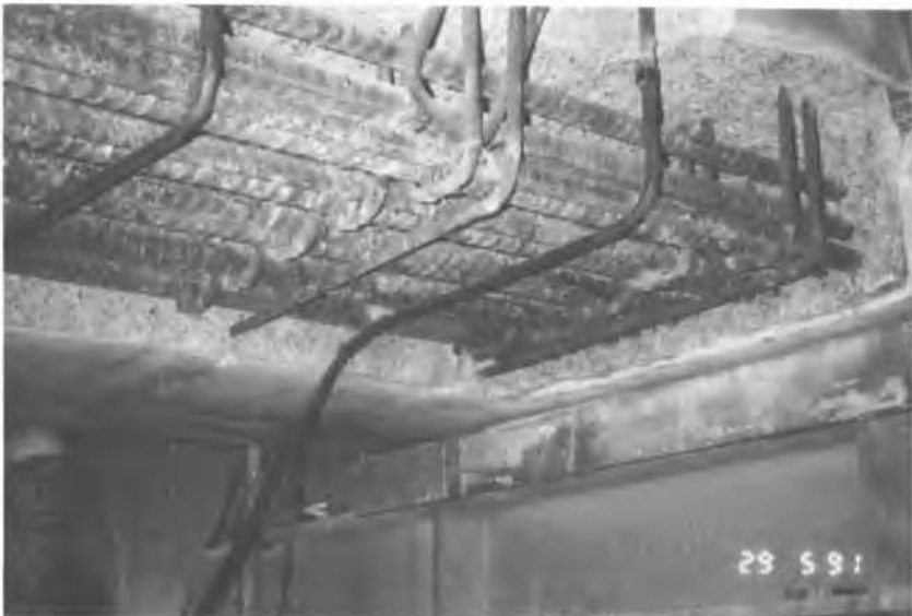
Fig. 1 Congested reinforcement in soffit
