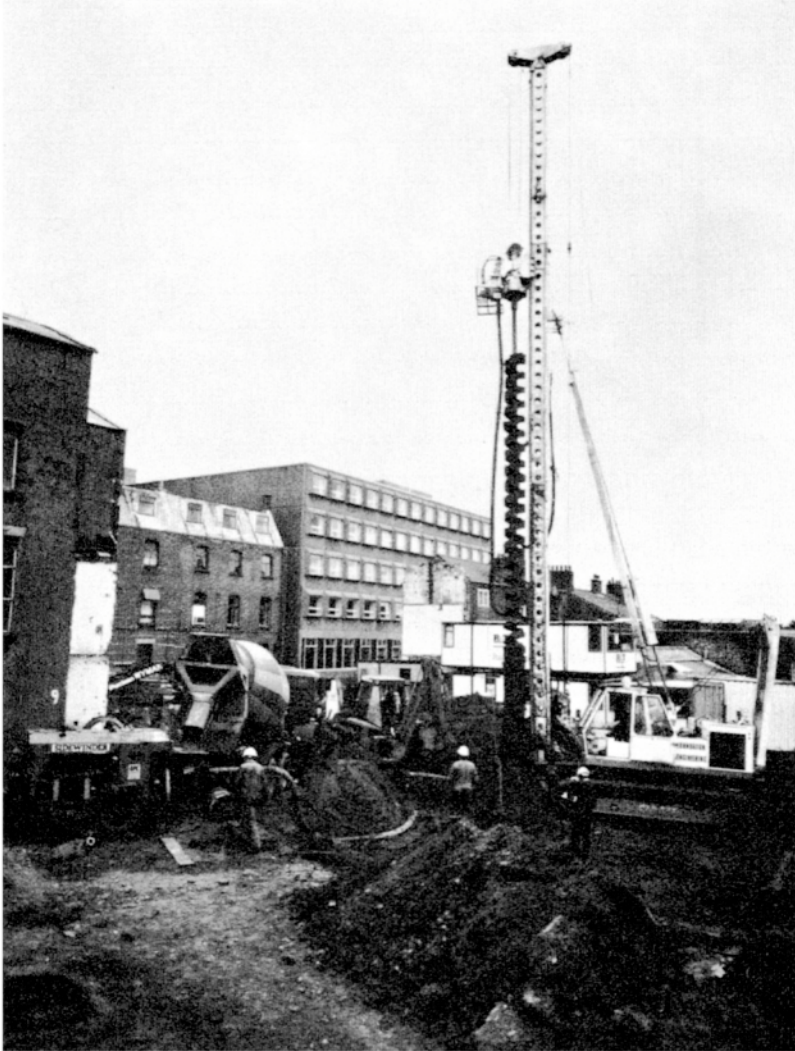
Figure 10.6 Supply to a continuous-flight auger (cfa) piling site. Courtesy Foundation Engineering Ltd
