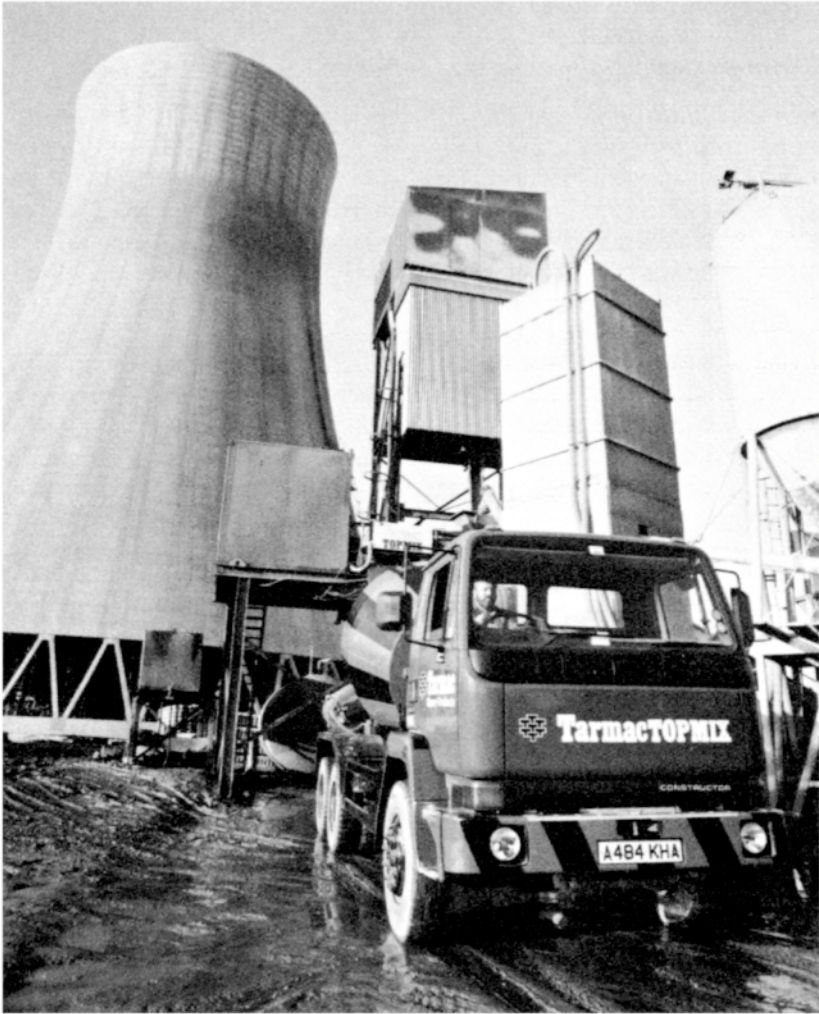
Figure 10.1 Transportable plant at a power station site. Courtesy Tarmac Topmix Ltd
