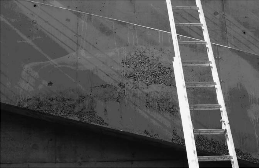
Figure 7.2 Honeycombs in monolithic spandrel beams placed integrally with deep, thin walls. This element was placed with a well-proportioned and adequately produced SCC mixture. These honeycombs developed because of excessive obstructions encountered during free fall into the formwork. The occurrence of honeycombing could have been reduced had the element been detailed in such a way that the top portion of the beam had been gradually chamfered (tapered) into the wall face. Courtesy of CTL Group.
