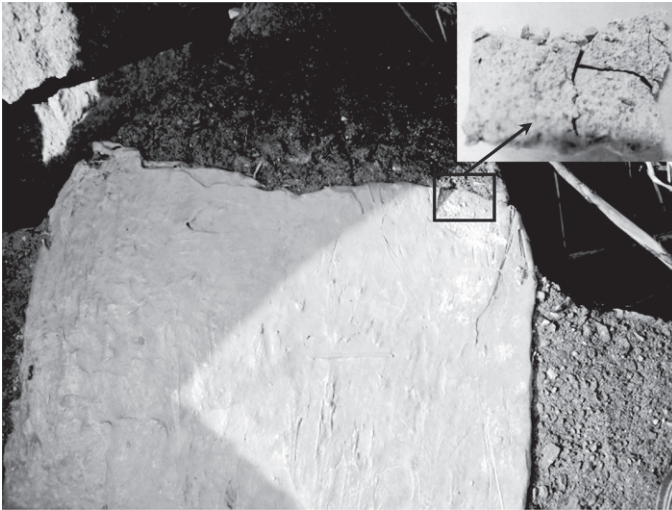
Figure 22.13 Examination of the bonding between AAM coating layer and OPC concrete after 180 days of exposure under marine tidal conditions.
