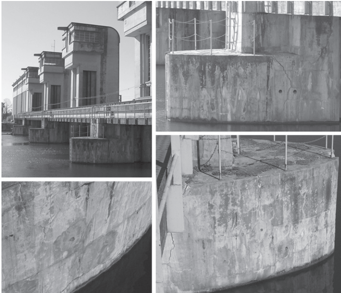
Figure 15.1 View of an ASR cracking pattern in a dam.
