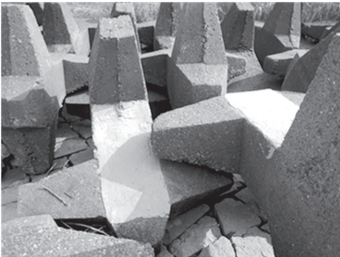
Figure 22.12 Hardened coatings on OPC concrete substrates after 180 days.
