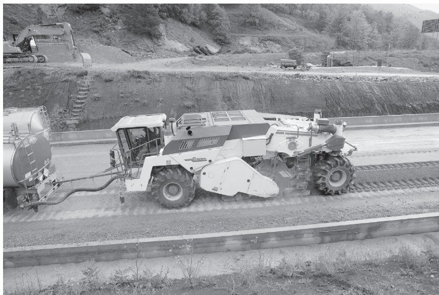
Figure 21.6 Photograph of surface mixing taking place at a site in India (courtesy of Wirtgen Group, 2014).
