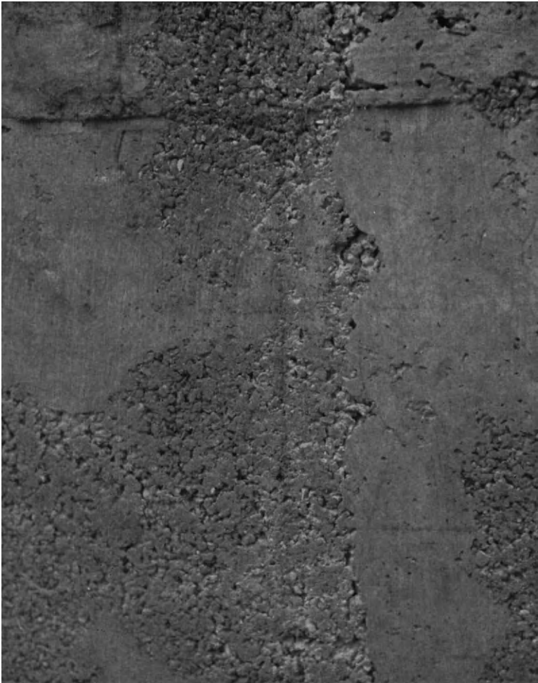
Plate 8. Poor compaction of workable concrete (Note nib where concrete has flowed between shutter joints)
