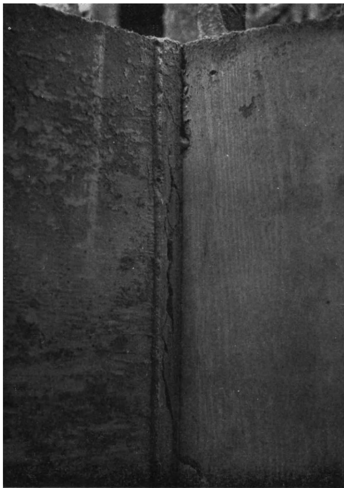
Plate 2. Drying shrinkage crack located at change of section.
