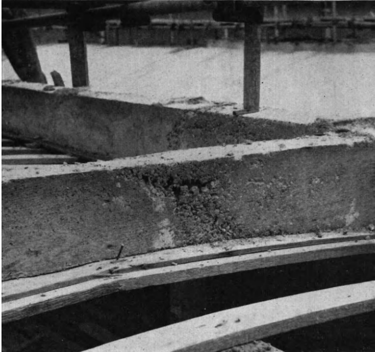
Plate 7. Faulty construction caused by poor compaction.
