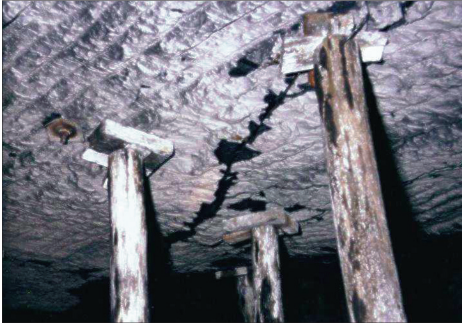
Figure 1. Example of a tension crack in the roof over a roadway
