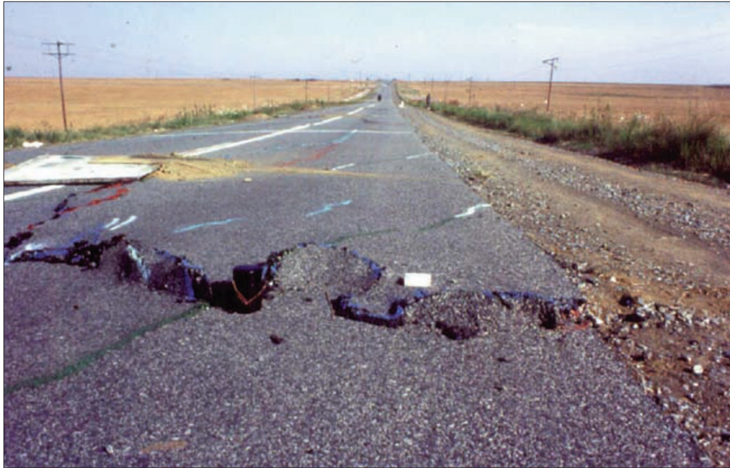
Figure 10. The compression ridge in the foreground is crossed at right-angles by an open tension crack. This is an illustration of a case where the one principal strain was compressive and the other one tensile. This shows that it may be an oversimplification to approach subsidence problems two-dimensionally; it is often necessary to consider the full three-dimensional impact of subsidence. (Photograph courtesy of EHR Schümann)
