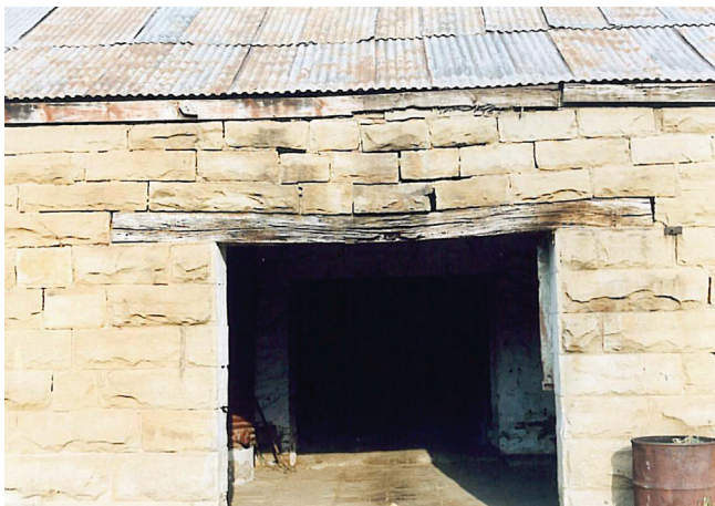
Figure 7. Stabilising effect of a timber lintel on bricks across a door opening
