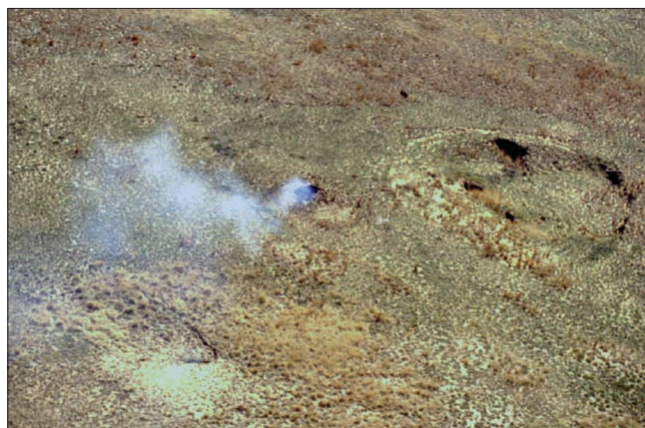
Figure 22. The depression on the right-hand side of the photograph was caused by the underground fire, indicated by the smoke coming out of the sinkhole
