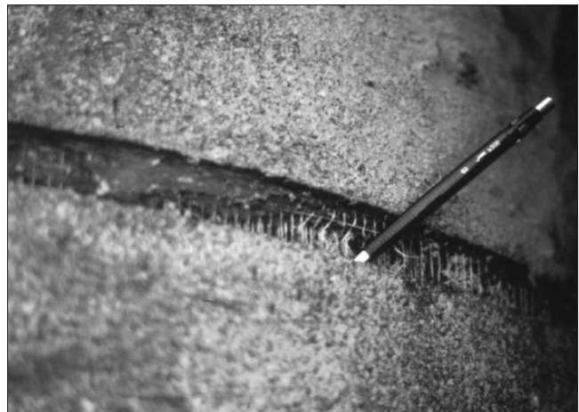
Figure 24. Even though the insulation material around the pipe was torn by the friction caused by horizontal displacement, the steel material of the pipe was not damaged
