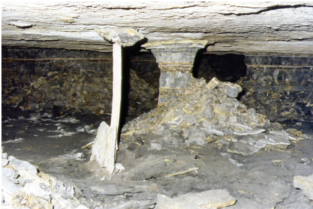
Figure 17. Example of a small pillar that has not failed because the load acting on it is less than the TAT load
