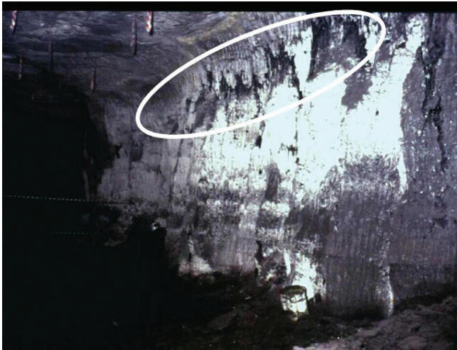
Figure 2(a). An example of ribside guttering, indicating that the vertical stress is in excess of the horizontal, or the k-ratio is less than unity
