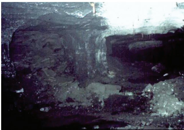
Figure 15. View of a well-designed snook system. The photograph was taken behind the last line of unmined pillars, just off the picture on the right. Note the line of snooks that are still standing, while the area behind them has goafed
