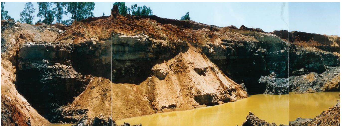
Figure 1. Collapse of 'softs' material extending to the pit floor because no bench between the 'softs' and 'hards' material was provided
