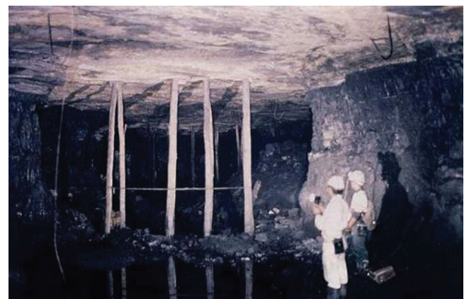
Figure 23. A timber breakerline installed in a pillar extraction section at high mining height. The effectiveness of such a breakerline is questionable
