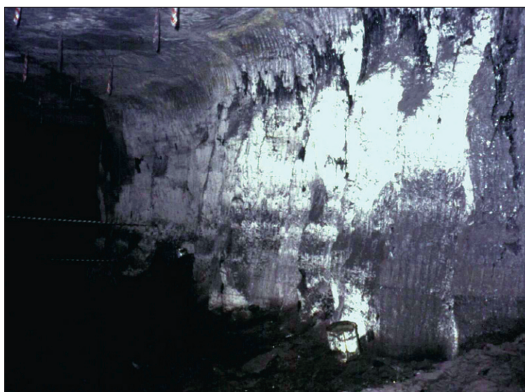
Figure 18. Sidewall guttering, indicating that the vertical stress on the pillar exceeds the horizontal stress
