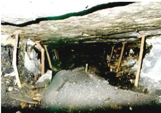
Figure 33. Example of floor heave in old workings
