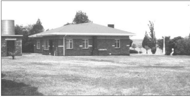
Figure 31. The Sasol Centre for Ground Conservation in Secunda, South Africa. The white markings on the walls indicate the floor elevation of the house before subsidence
