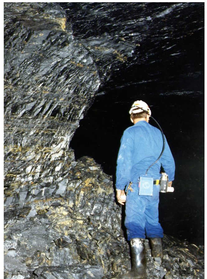
Figure 7. Severe scaling of a pillar in the Vaal Basin. Note that the roof is still intact
