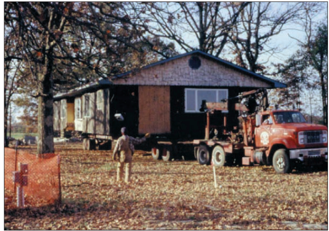
Figure 33. A house in the USA being removed to a stable position prior to undermining (Photograph courtesy of Robert A Bauer)
