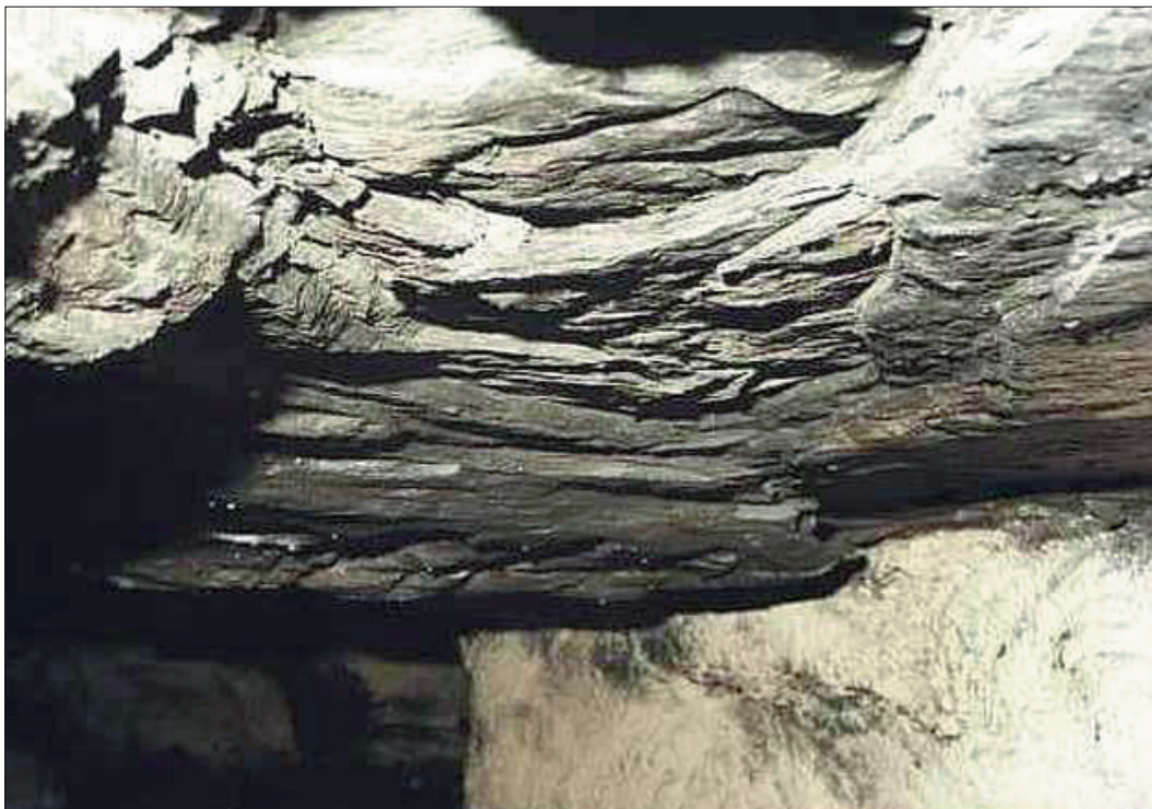
Figure 2. Over-thrusting in the roof caused by high horizontal stress
