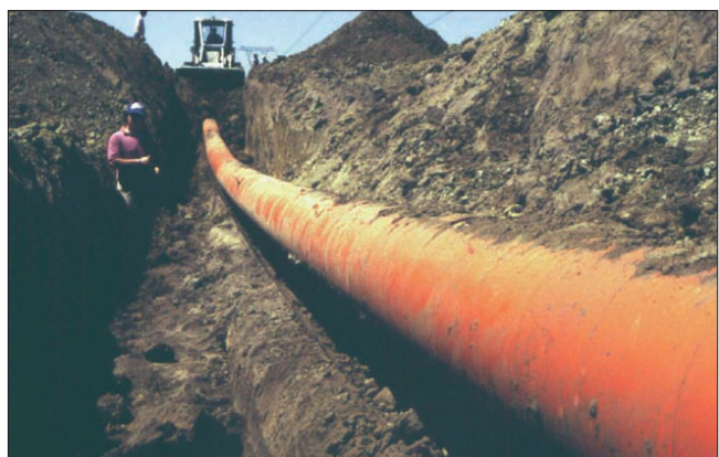
Figure 25. This pipe lifted clear off the ground surface after being uncovered
