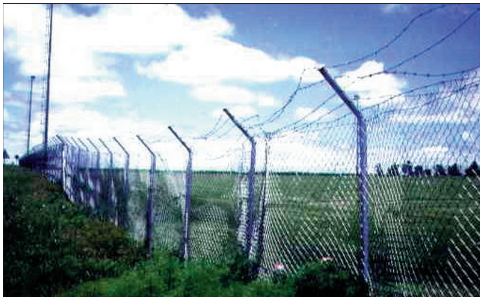
Figure 25. The slack in the fence is a good indication of the position of the compressive zone in a subsidence trough
