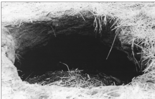
Figure 18. A freshly collapsed sub-surface erosion pothole, ballooning out below the surface. The diameter of the hole on the surface is about 50 cm
