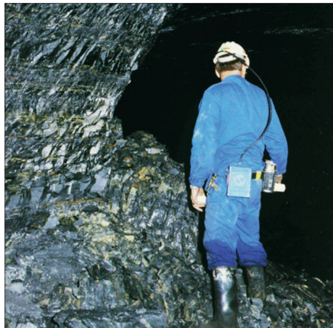
Figure 16. Severe pillar scaling, resulting in a concave-shaped pillar
