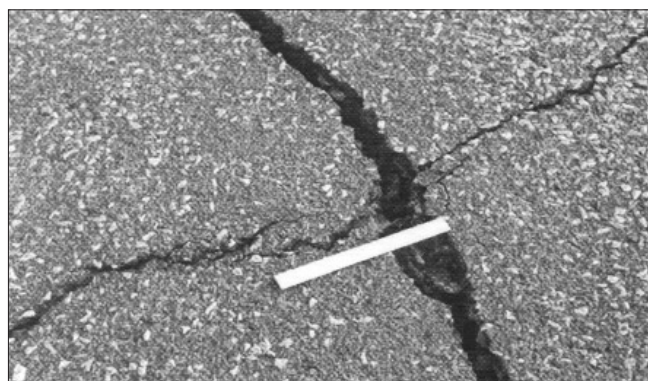
Figure 26. Cracks on the road surface caused by tensile strain. Note that in this case, both of the principal strains were tensile
