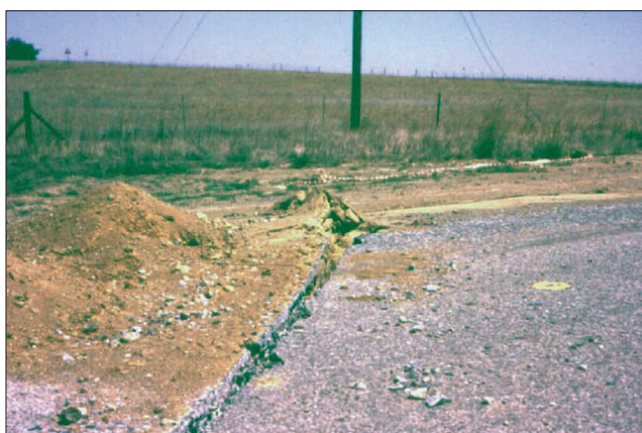
Figure 28. The slot in the photograph was originally 30 cm wide. Compressive strain caused by undermining reduced the width to 10 cm. Note the ridge on the road shoulder in the background, where no slot was provided. If the slot had not been cut in the road, a ridge of the same height would have developed on the road
