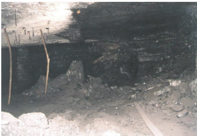
Figure 20. A timber ‘policeman’ providing indication of a sagging roof. This method is not always effective at shallow depth
