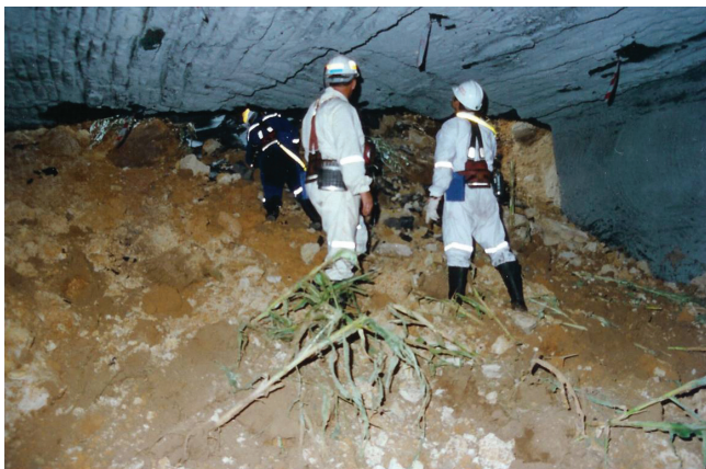
Figure 6. Sudden failure of incompetent layers at shallow depth
