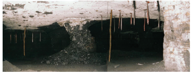
Figure 14. Small pillar snooks showing no signs of load
