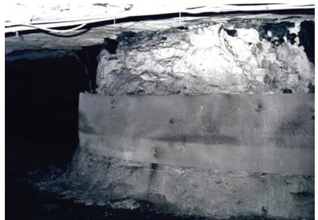
Figure 35. An old pillar that has been stabilized by wrapping with discarded conveyor belting
