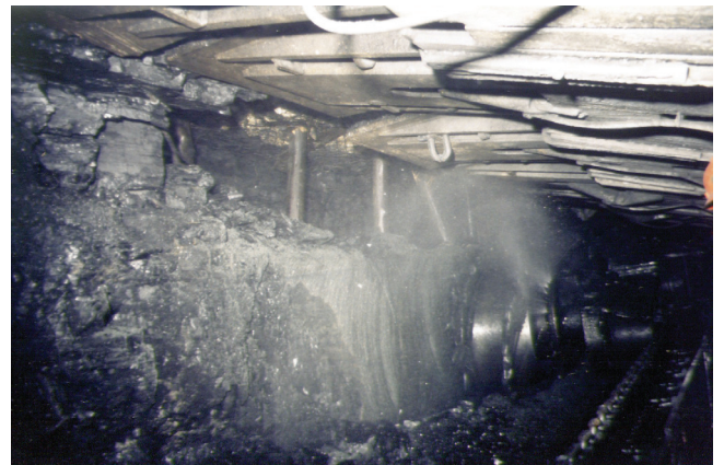
Figure 24. Mining through the filled excavation in an area where the second stage filling was not done successfully. If the timbers had not been installed, roof falls would probably have occurred
