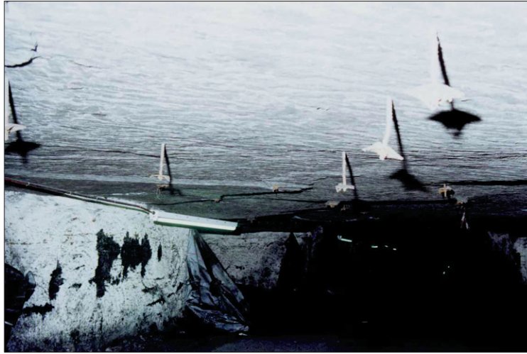
Figure 3. Illustration of a typical fall indicating a lack of pre-tension on the bolts and excessive spacing
