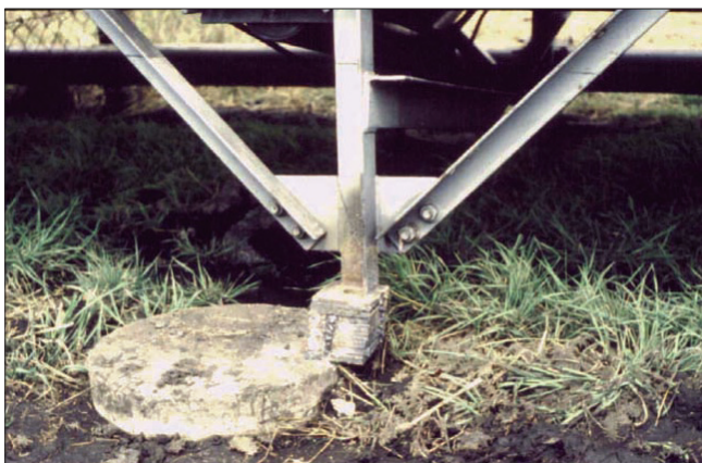
Figure 23. Horizontal displacement of the ground surface is the most important subsidence element that could affect the operation of a conveyor belt. The bolt, holding the leg of the structure to the foundation block, should be cut to allow the belt to maintain itself in a straight line
