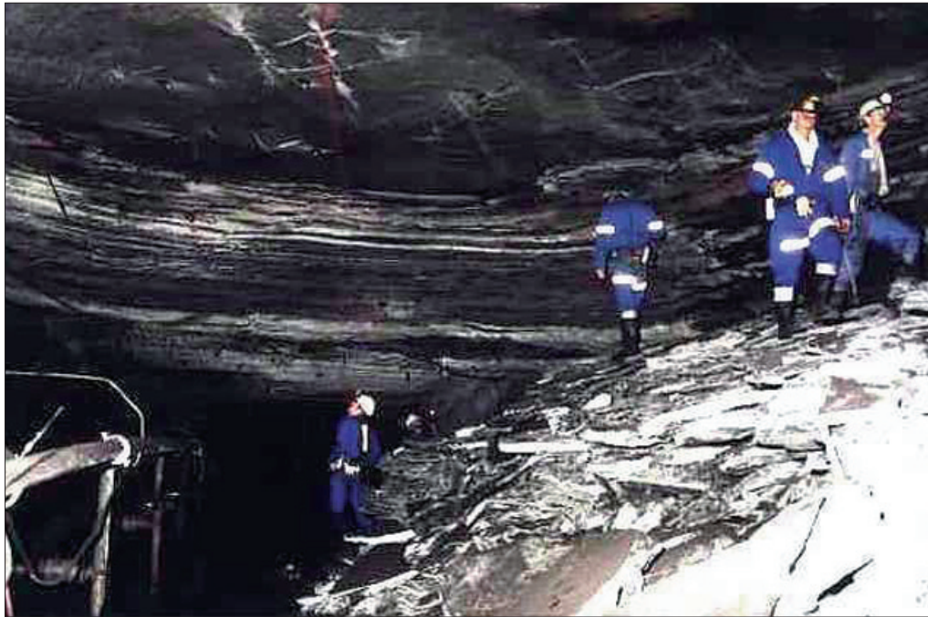
Figure 5. Example of a roof that fell out higher than the length of the bolts. The roof under which the people are seen, was re-supported even though the bolts cannot be clearly seen in the photograph
