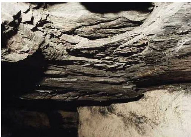
Figure 2(b). An example of roof guttering, indicating that the horizontal stress is greater than the vertical, or that the k-ratio is greater than unity
