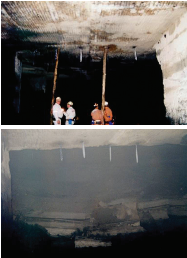
Figure 24. A roofbolt breakerline before the goaf (top picture) and the same one after the goaf (bottom picture). The chevron tape hanging from the roof indicates the positions of the roofbolts. Note the ‘policeman sticks’ in the upper picture
