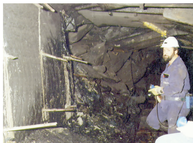
Figure 17. This face has been stabilized by installing wooden dowels in the hitherto sound area close to the face break in the background
