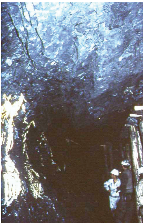
Figure 15. The light coloured material oozing out of the face is polyurethane that was used to stabilize a standing face to prevent a possible face break. The fractures can be seen in the top left corner of the photograph. The timbers on the right-hand side of the photograph were installed under the shield tips, another precaution
