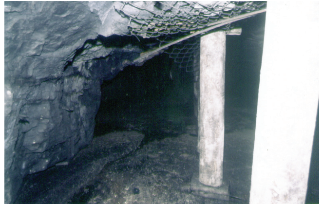
Figure 23. Second stage filling flowing into the excavation after the timbers had been installed. The timbers are installed on foot boards to prevent them punching into the fill
