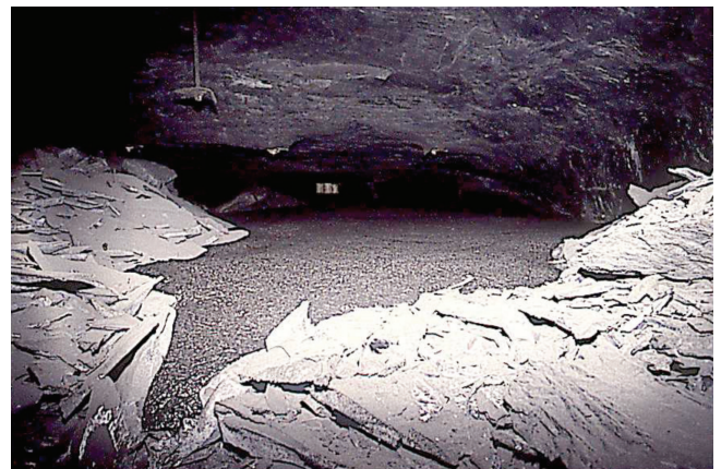
Figure 16. Filling with fine coal at Sigma Colliery. Note the scaling debris from the pillars on the floor and the largely intact roof
