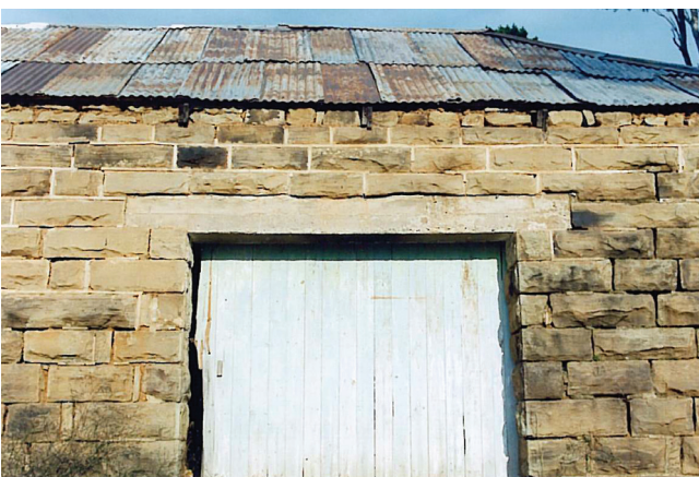
Figure 8 Enhanced stabilizing effect of a concrete lintel on bricks across a door opening
