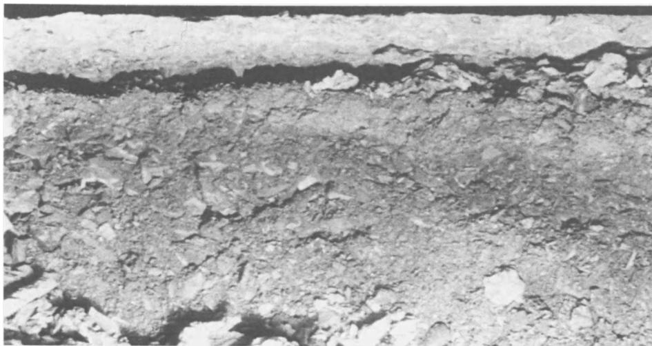
Plate 5. Disintegration of Concrete Floor Slab due to Sulphate in underlying Burnt Minestone.
