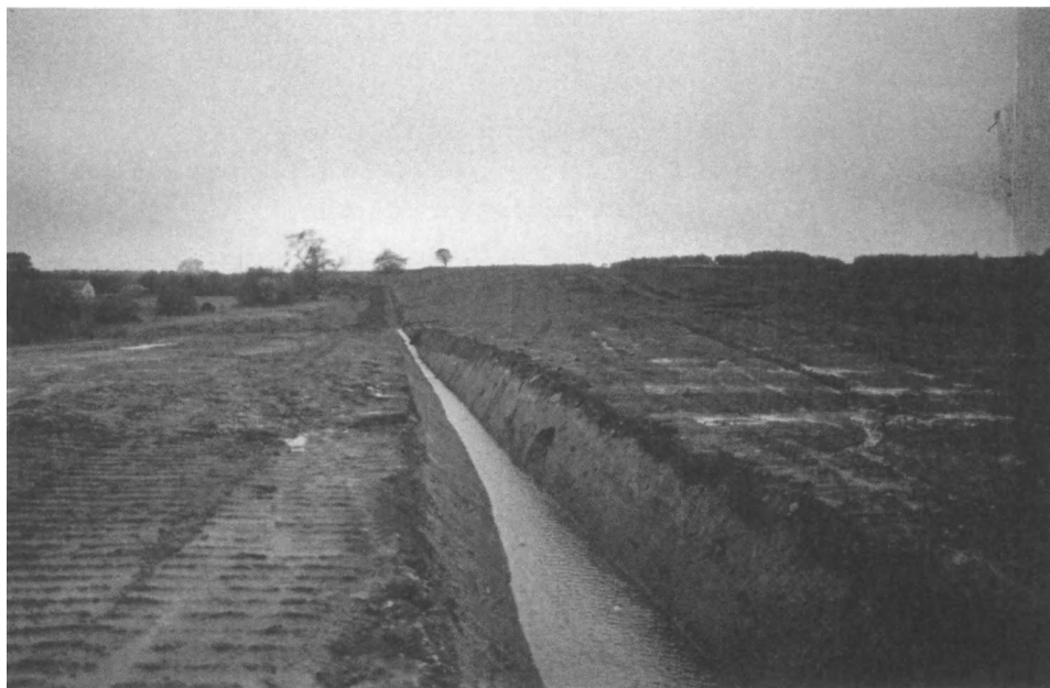
Figure 8 Completion of phase 1 coal recovery/regrading at Meikle Earnock tip, Hamilton. Phase 2 will include the cultivation of the main site area to the right of the ditch which, in turn, will be piped and gravel backfilled.
