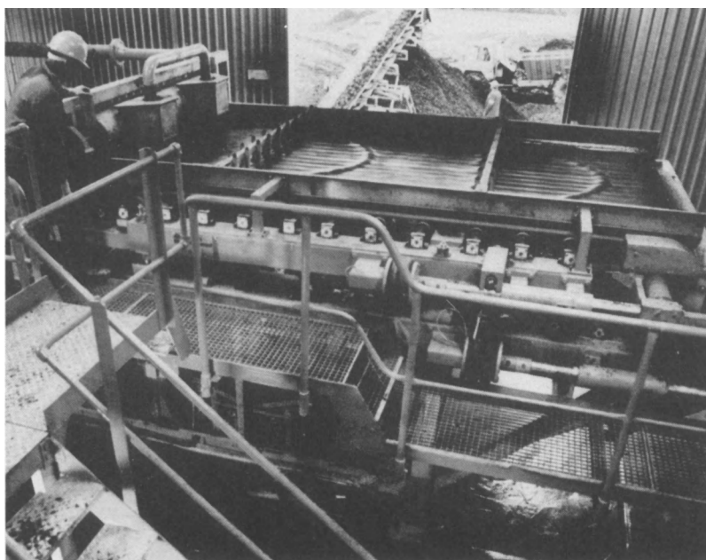
Figure 2. Andritz CPF in operation in North-East England.
