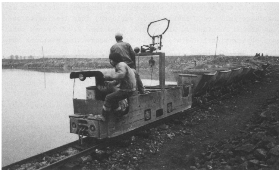
Fig. 3. Land reclamation by dumping dirt into the subsidence pit accumulated with water.
