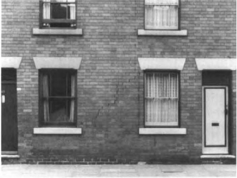
Photograph 3.1: Example of external structural damage caused by mining subsidence (source: British Coal)
