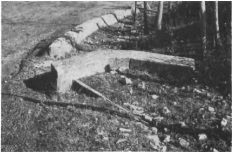
Photograph 15.5: This drainage system is completely blocked by silt. Regular inspection and clearance is essential (source: Welsh Development Agency)
