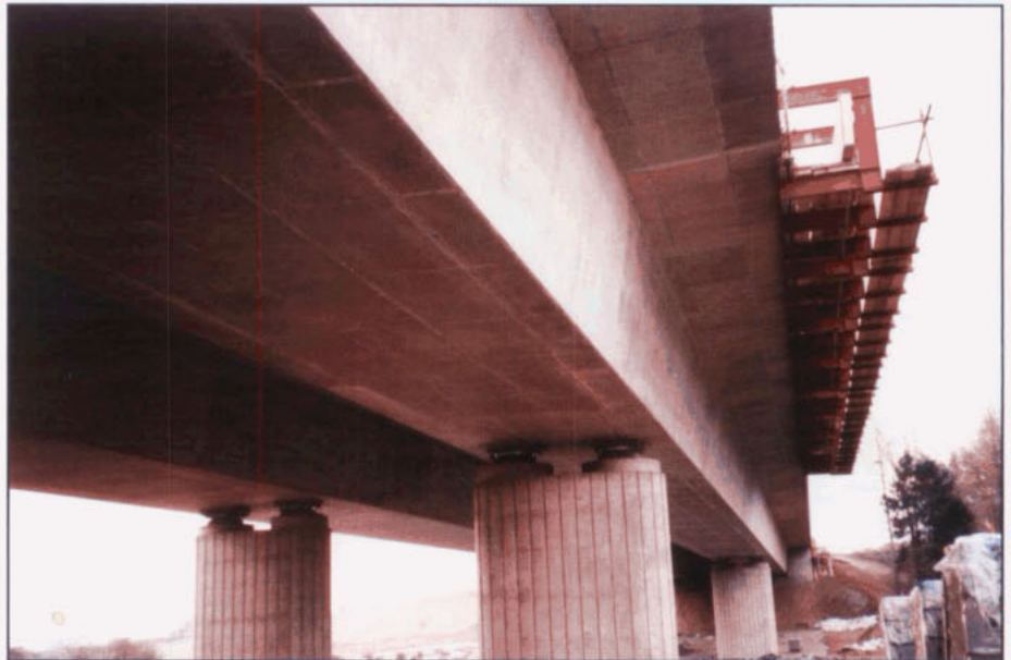
Figure 9 Traveller being used for the construction of a deck cantilever and stringcourse
