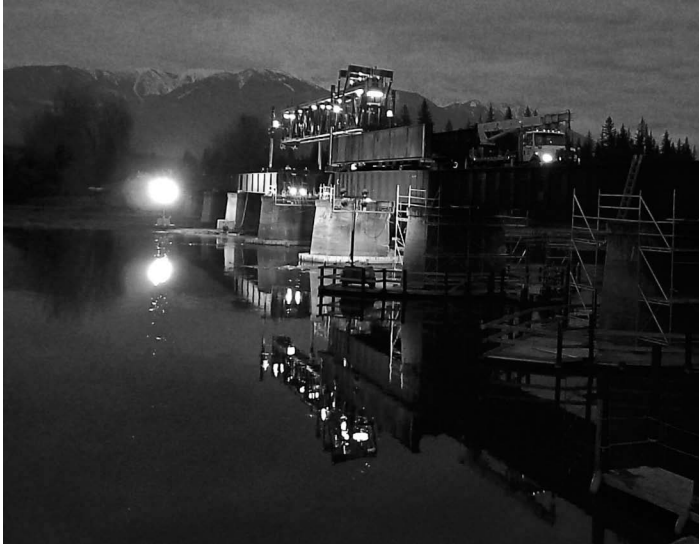
FIGURE 11.22 Span erection with single-span movable frame. (Courtesy of the Author, Canadian Pacific Engineering, Calgary, AB, Canada.)
