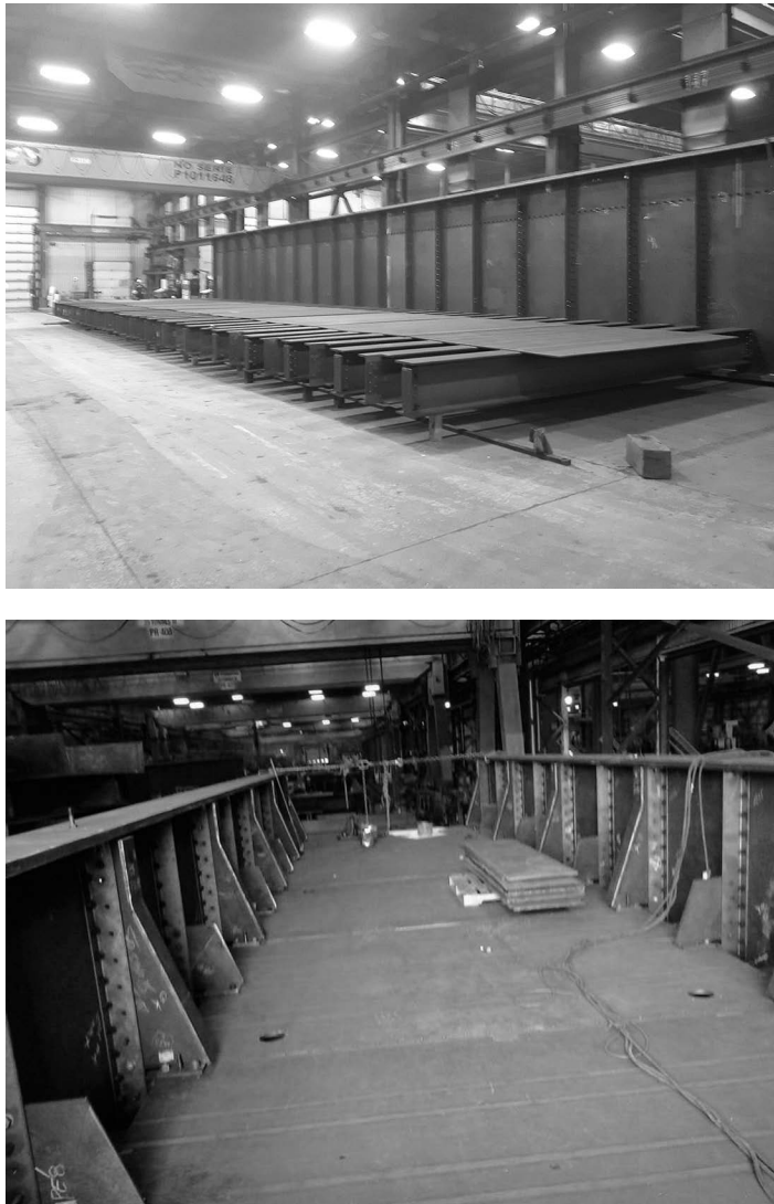
FIGURE 10.9 (a) Complete shop assembly of a BTPG span (one girder). (b) Complete shop assembly of a BTPG span (two girders). ((a) Courtesy of F. Mathieu, SGS Inc., Quebec City, QC, Canada; (b) Courtesy of the author, Calgary, AB, Canada.)
