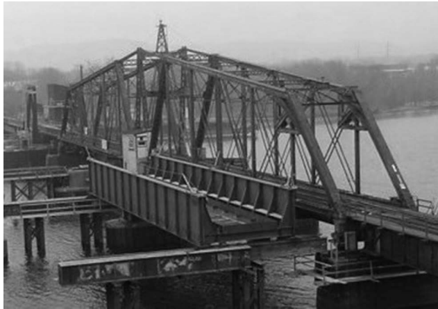
FIGURE 11.13 Nonintrusive falsework for lateral rolling erection of new BTPG spans. (Courtesy of the author, Canadian Pacific Engineering, Calgary, AB, Canada.)
