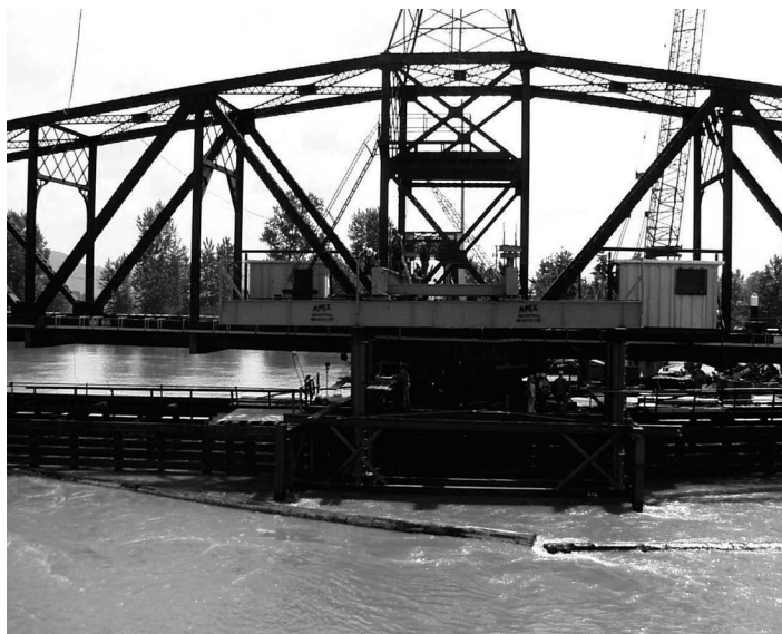
FIGURE 11.30 Frame for horizontal moving of truss. (Courtesy of the Author, Canadian Pacific Engineering, Calgary, AB, Canada.)
