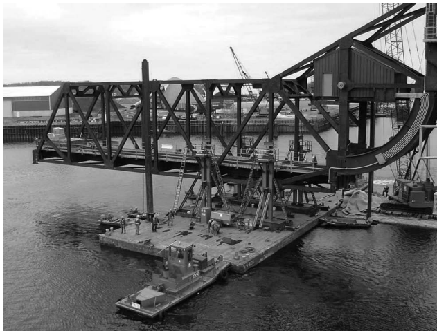
FIGURE 11.16 Superstructure supported on falsework on barge. (Courtesy of the Author, Canadian Pacific Engineering, Calgary, AB, Canada.)
