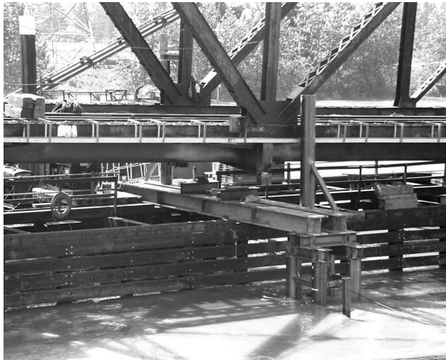
FIGURE 11.12 Nonintrusive emergency falsework. (Courtesy of the Author, Canadian Pacific Engineering, Calgary, AB, Canada.)
