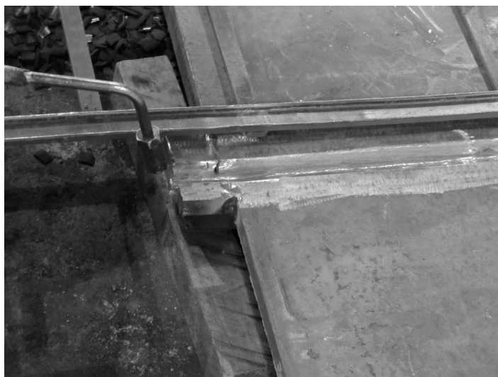
FIGURE 10.28 Run-on/run-off pieces for SAW butt weld. (Courtesy of Dr. K. Frank, Hirschfeld Industries, Austin, TX, USA. With permission.)
