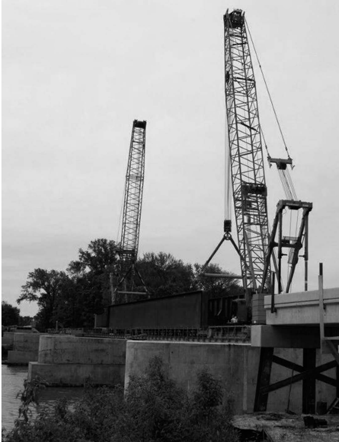
FIGURE 11.29 Erection with tandem cranes. (Courtesy of D. Ostby, Koppers Railroad Structures, Madison, WI, USA. With permission.)
