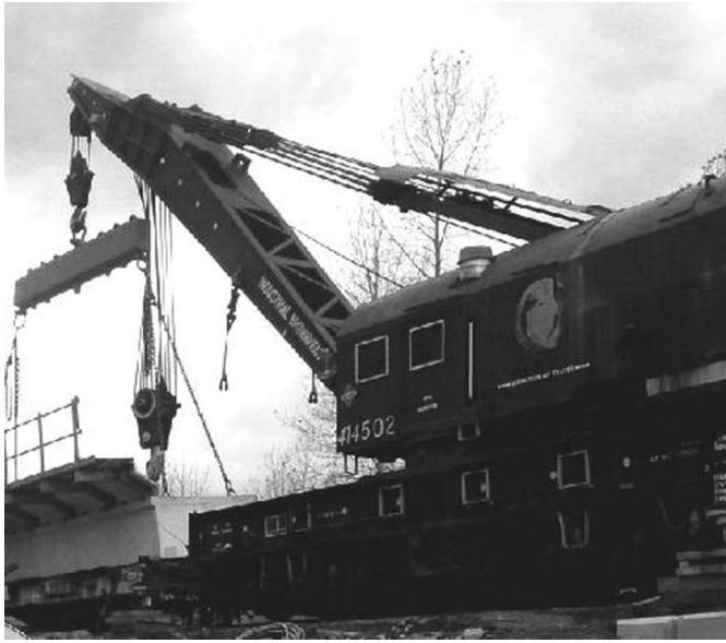
FIGURE 11.10 Locomotive crane lifting short span. (Courtesy of the Author, Canadian Pacific Engineering, Calgary, AB, Canada.)
