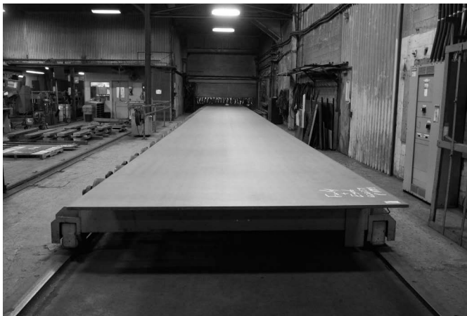
FIGURE 10.8 Surface preparation to SSPC specification SP6. (Courtesy of Y. Martin, Canam Bridges Inc., St. Foy, QC, Canada. With permission.)
