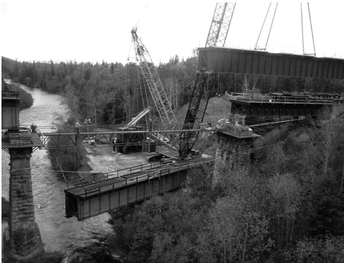
FIGURE 11.6 Crawler crane lifting new DPG span onto existing rehabilitated substructures. (Courtesy of the Author, Canadian Pacific Engineering, Calgary, AB, Canada.)
