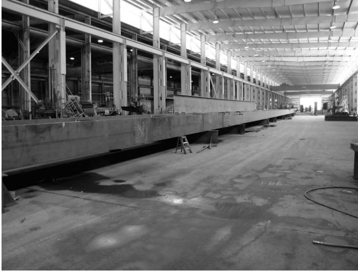
FIGURE 10.3 Layout of a long plate girder. (Courtesy of Dr. K. Frank, Hirschfeld Industries, Austin, TX, USA. With Permission.)
