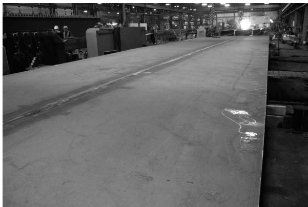
FIGURE 10.17 Web plate butt weld joint. (Courtesy of Y. Martin Canam Bridges Inc., St. Foy, QC, Canada. With permission.)
