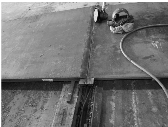
FIGURE 10.12 Plate preparation for groove welding. (Courtesy of Dr. K. Frank, Hirschfeld Industries, Austin, TX, USA. With permission.)
