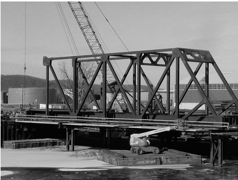
FIGURE 11.1 Stick-building of truss span on falsework at site assembly yard. (Courtesy of the Author, Canadian Pacific Engineering, Calgary, AB, Canada.)
