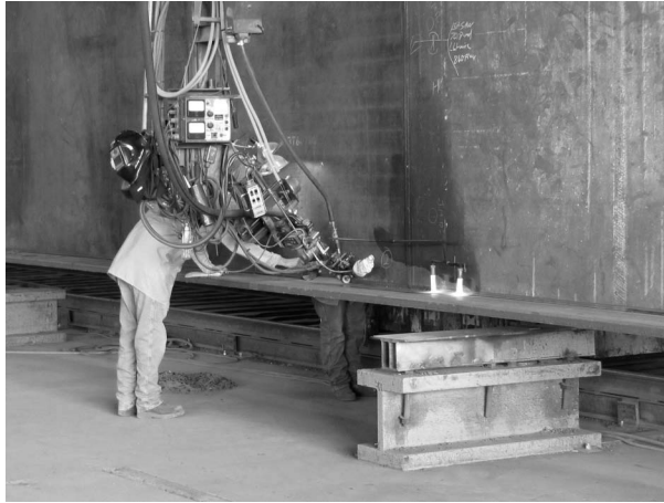
FIGURE 10.15 SAW flange-to-web welding with girder in vertical position. (Courtesy of Dr. K. Frank, Hirschfeld Industries, Austin, TX, USA. With permission.)
