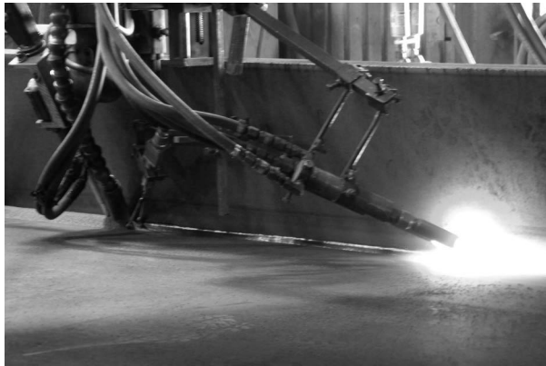
FIGURE 10.16 SAW flange-to-web welding with girder in horizontal position. (Courtesy of Y. Martin, Canam Bridges Inc., St. Foy, QC, Canada. With permission.)
