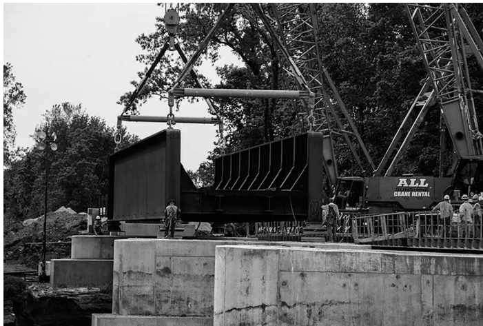
FIGURE 11.28 Erection of complete span. (Courtesy of D. Ostby, Koppers Railroad Structures, Madison, WI, USA. With permission.)
