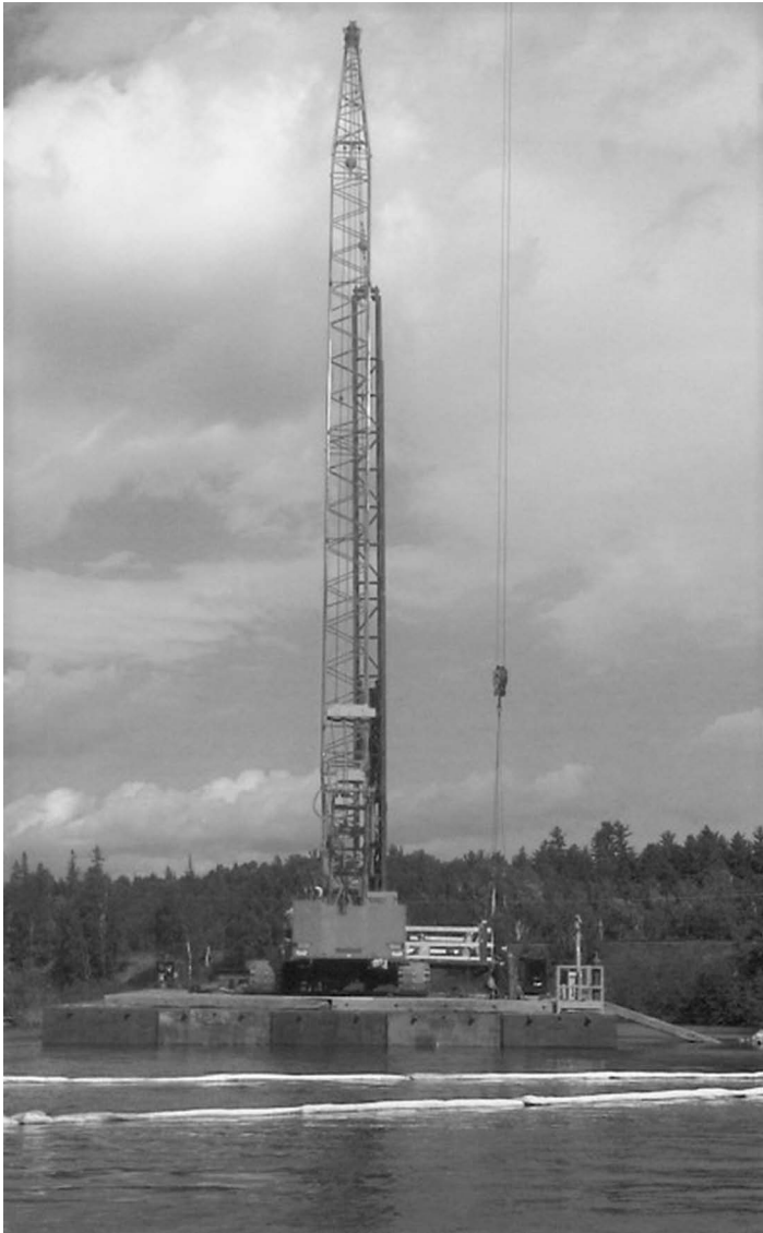
FIGURE 11.17 Crawler crane on barge for pile driving. (Courtesy of the Author, Canadian Pacific Engineering, Calgary, AB, Canada.)
