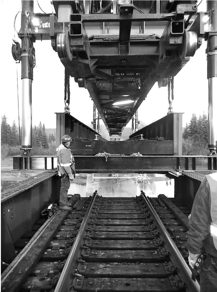
FIGURE 11.19 Sequential replacement of steel spans using a movable frame. (Courtesy of the Author, Canadian Pacific Engineering, Calgary, AB, Canada.)
