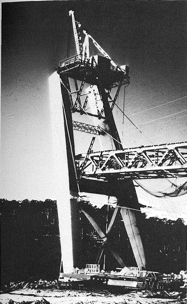
FIGURE 8.29 Batman Bridge, climbing crane on pylon. (Courtesy of Department of Public Works, Tasmania, from reference 18.)
