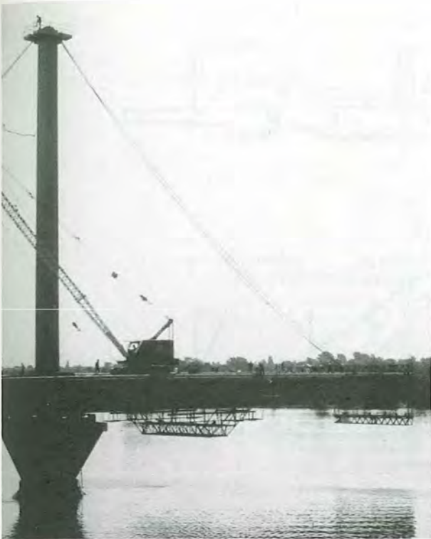
FIGURE 8.22 Papineau-Leblanc Bridge, tower and inside stay erection. (Courtesy of Paul Marquis, Gendron Lefebvre and Associates.)
