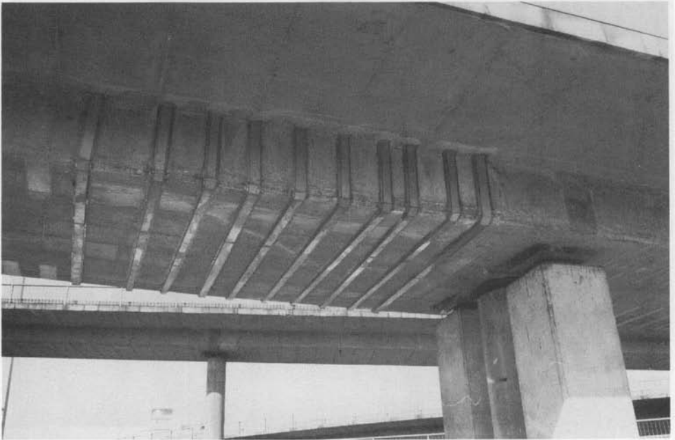
Figure 6.5 Stainless steel sheathing to cables shown in Fig 6.4 grout-filled to protect cables against corrosion (courtesy of S Roux)
