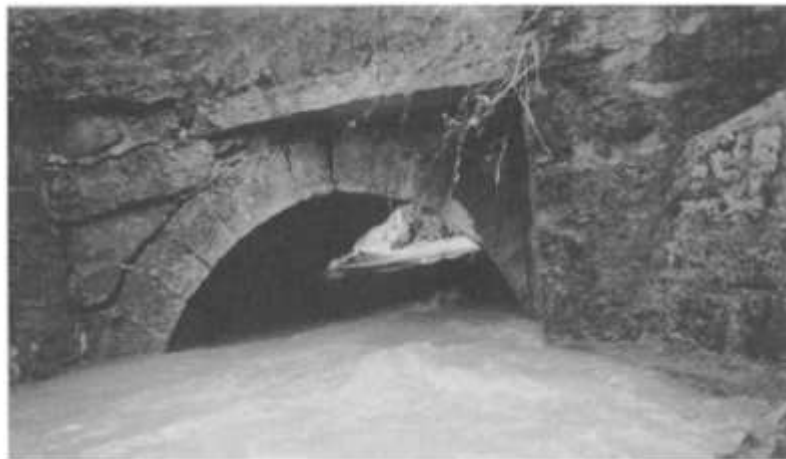
Fig. 1.8 This 2.06 m span bridge at Polgooth, Cornwall, is reported to have severely obstructed the stream and thus contributed to severe flooding in the village in November 1997. The bridge itself exhibits separation of the upstream arch ring; undermining of the foundations was suspected. It also suffered a partial collapse downstream, and is to be replaced by a reinforced concrete deck-type bridge. This example serves as a reminder that small bridges must also be designed with care. (Reproduced by permission of Cornwall County Council)
