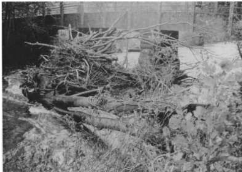
Fig. 1.11 Debris can be a particular problem in forested areas, as illustrated here by Whetcombe Barton Bridge on the River Teign, Devon, in 1960. The approximate flood level was at the bottom rail of the parapet. (Reproduced by permission of the Environment Agency)
