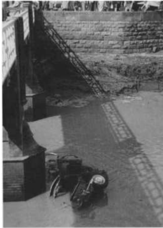
Fig. 1.10 Even the performance of a well-designed bridge can be adversely affected by unexpected flood debris; Ham Footbridge, River Sid, Sidmouth in July 1968. (Reproduced by permission of Hayes Studio, Sidmouth)
