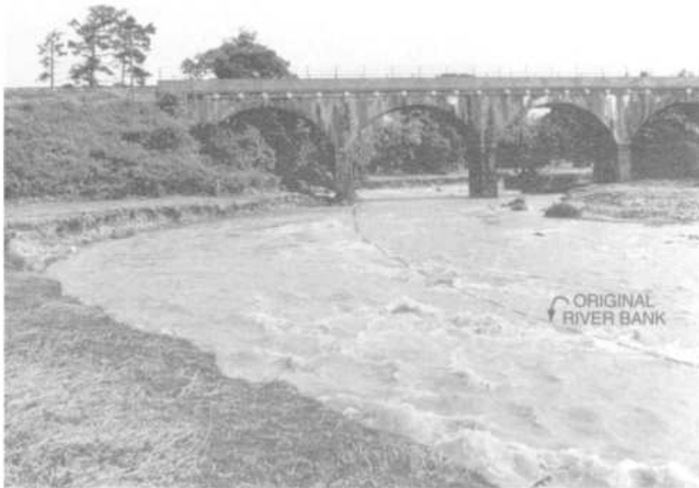
Fig. 1.6 Lateral erosion downstream of the railway viaduct at Fenny Bridges, Devon, in July 1968. The line of the original river bank is shown by the dashes. Changes of this type can significantly alter the angle at which the flow hits the piers and thus affect scour depths. (Reproduced by permission of the Environment Agency)
