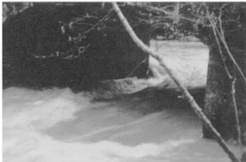
Fig. 2.8 Type 6 supercritical flow in the opening and downstream channel. This bridge is eccentric to the channel so there is a considerable flow along the upstream face of the right hand abutment (on the left in the photo). This pushes the jet towards the left abutment, narrows the vena contracta, and results in high velocities (see Fig. 7.11 ).
