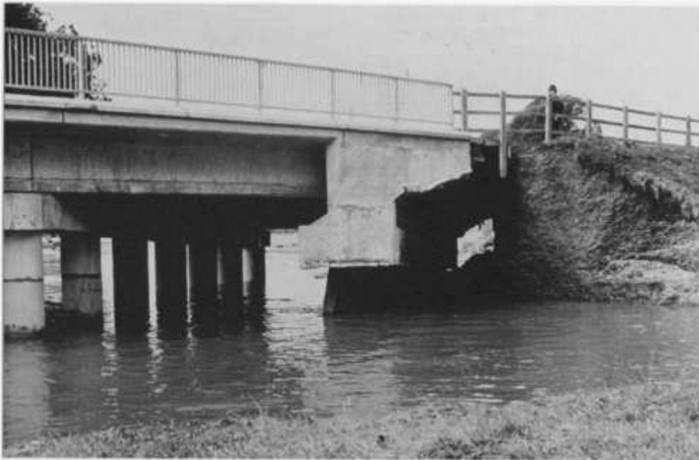
Fig. 8.2 Bank erosion at Stoneyford Bridge, Honiton, July 1968. (Reproduced by permission of the Environment Agency)
