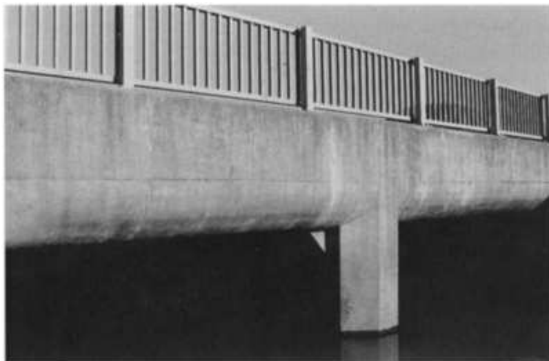
Fig. 7.1 A modern bridge at Plympton, Devon, having a rounded soffit and a pier with chamfers.
