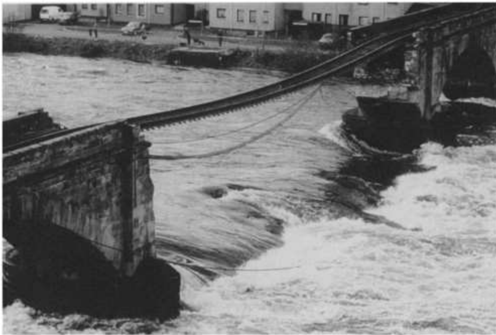
Fig. 1.9 Part of the viaduct over the River Ness, which collapsed in February 1989. Scour was suspected to be the cause. (Reproduced by permission of John Paul Photography, Inverness)
