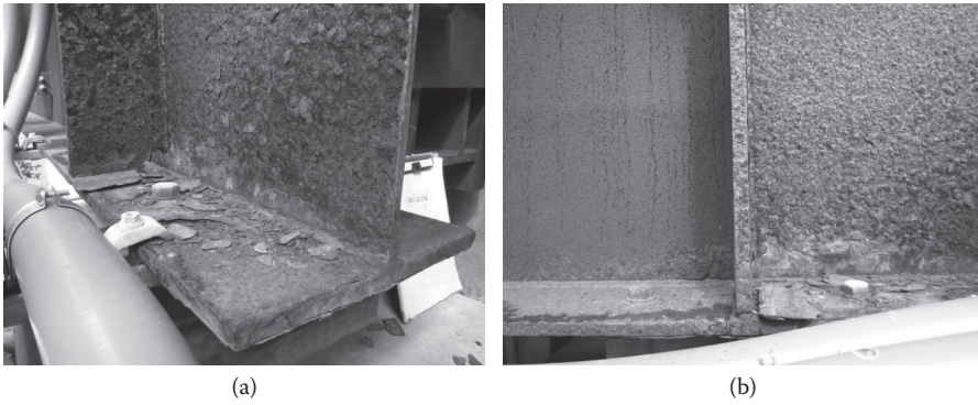
FIGURE 17.5 Unfavorable corrosion state: (a) view from girder end, (b) side view.
