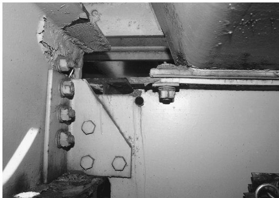
FIGURE 19.6 View of floorbeam of Throg's Neck Bridge in New York showing crack in the cope that has been repaired by drilling a stop hole. The crack is caused by incompatibility between the curvature of the superstructure and the orthotropic steel deck that is bolted onto the floorbeams.
