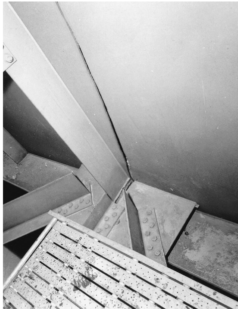
FIGURE 19.1 View of cracked girder of Lafayette Street Bridge in Minneapolis showing fatigue crack originating from backing bars and lack of fusion on the weld attaching the lateral bracing attachment plate to the web and to the transverse stiffener.
