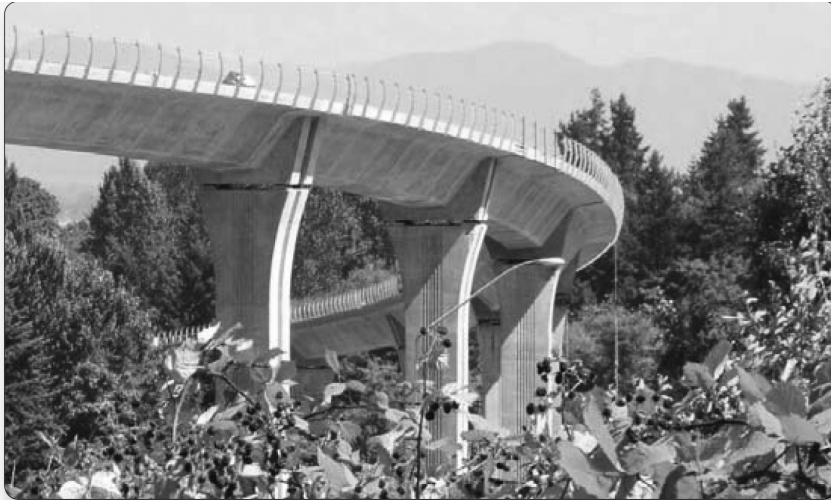
FIGURE 3.2 A conceptual engineering study for the Seattle LRT viaduct produced a design that both reduced cost and improved appearance compared to a standard design. (From AASHTO, Bridge Aesthetics Sourcebook , American Association of State Highway and Transportation Officials, Washington, DC, 2010. With permission.)
