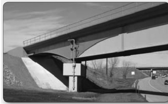
FIGURE 3.24 This drainage system and blocky pier clash with an otherwise attractive overall aesthetic scheme. Union Pacific Railroad Bridge over I-25, Castle Rock, Colorado. (From AASHTO, Bridge Aesthetics Sourcebook , American Association of State Highway and Transportation Officials, Washington, DC, 2010. With permission.)
