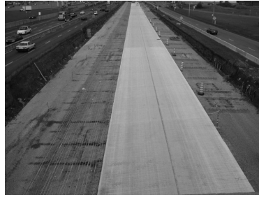
FIGURE 16.26 Reinforcement of the bridge deck slab and barrier walls, Val-Alain Bridge.(From ISIS, Design Manual 3: Reinforcing Concrete Structures with Fibre Reinforced Polymers . ISIS Canada, Intelligent Sensing for Innovative Structures, A Canadian Network of Centres of Excellence, University of Manitoba, Winnipeg, Manitoba, Canada, 2007a. With permission.)
