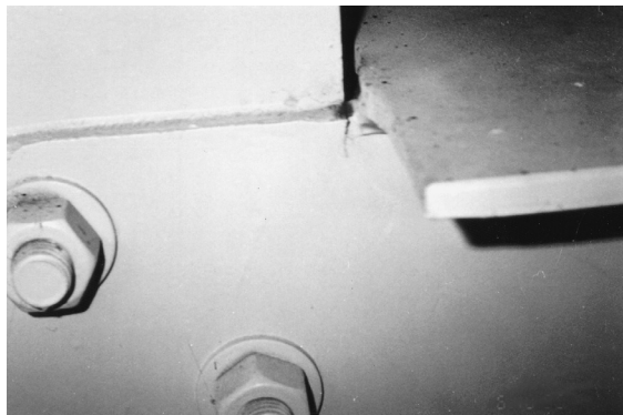
FIGURE 19.9 Close-up view of a crack originating at the termination of a flange on a floorbeam with a “simple” connection to an attachment plate in the Dresbach Bridge in Minnesota. The crack is an indication of an end moment in the simple connection that is not predicted in design.
