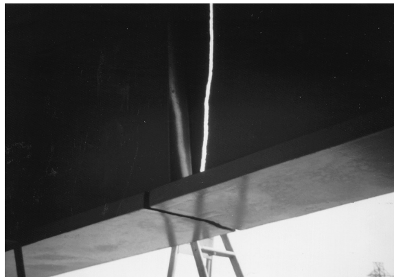
FIGURE 19.3 View of cracked girder of I-79 Bridge at Neville Island in Pittsburgh as an example of a bridge that is sufficiently redundant to avoid collapse despite a fracture of the tension flange and the web.
