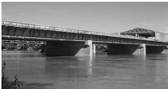
FIGURE 16.22 The Taylor Bridge, in Headingley, Manitoba, during construction. (From ISIS, Design Manual 3: Reinforcing Concrete Structures with Fibre Reinforced Polymers . ISIS Canada, Intelligent Sensing for Innovative Structures, A Canadian Network of Centres of Excellence, University of Manitoba, Winnipeg, Manitoba, Canada, 2007a. With permission.)
