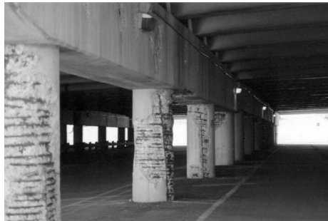
FIGURE 16.12 Deteriorated concrete columns.
