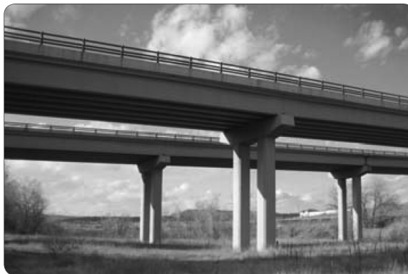
FIGURE 3.19 The substructure for this high-level crossing with slender piers is virtually transparent. Meadows Parkway over Plum Creek, Castle Rock, Colorado (Sourcebook 3.6). (From AASHTO, Bridge Aesthetics Sourcebook , American Association of State Highway and Transportation Officials, Washington, DC, 2010. With permission.)
