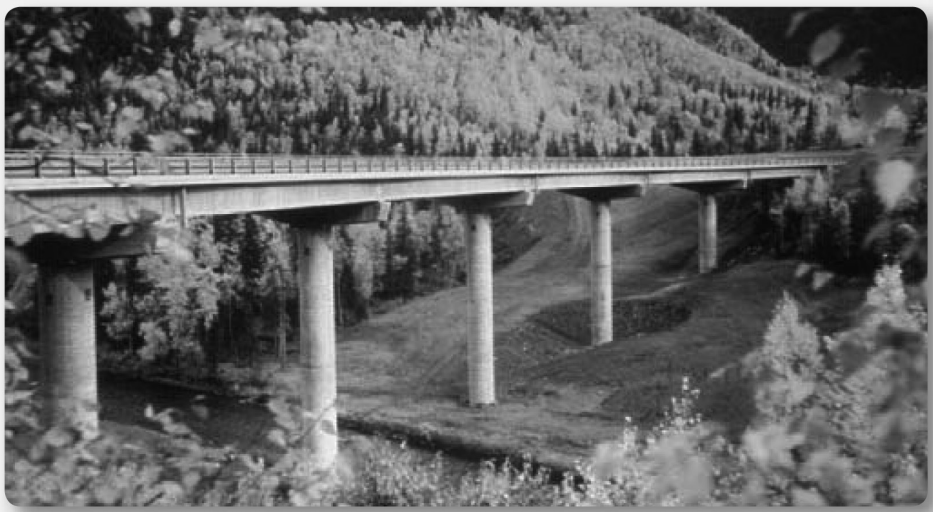
FIGURE 3.1 Often simply paying attention to proportions and details can result in an attractive bridge with no increase in cost. Canyon Creek Bridge, Anchorage, Alaska. (From AASHTO, Bridge Aesthetics Sourcebook , American Association of State Highway and Transportation Officials, Washington, DC, 2010. With permission.)
