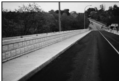
FIGURE 16.27 Deck rehabilitation of Glendale Avenue Bridge.(From ISIS, Design Manual 3: Reinforcing Concrete Structures with Fibre Reinforced Polymers . ISIS Canada, Intelligent Sensing for Innovative Structures, A Canadian Network of Centres of Excellence, University of Manitoba, Winnipeg, Manitoba, Canada, 2007a. With permission.)
