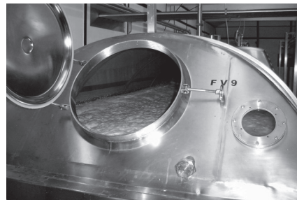
Enclosed fermentation vessel at Jennings' Brewery.
