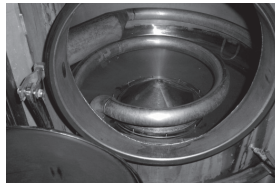
Detail of the gas heating rings in the kettle at Nottingham Brewery.
