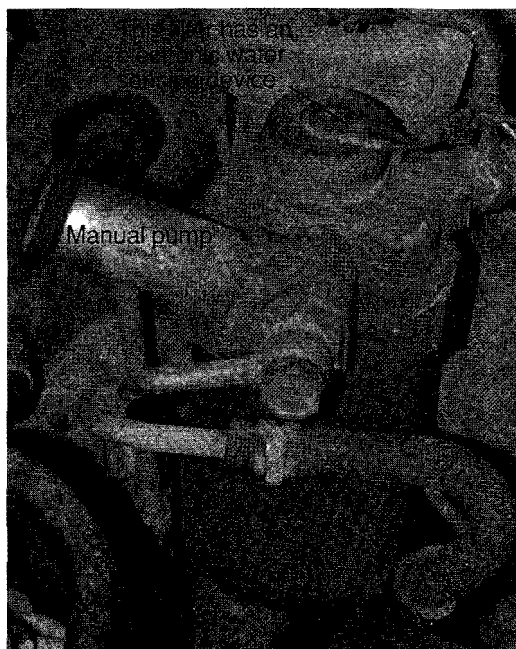
Figure 9-9. Manual fuel pump on a filter.
