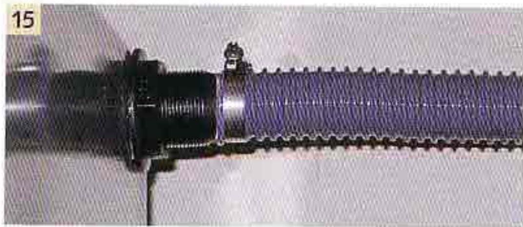
15 Hose (4 centimetres) for venting/draining the bottle locker. Any gas leaking from either the bottle or the pipes runs out to the transom.
