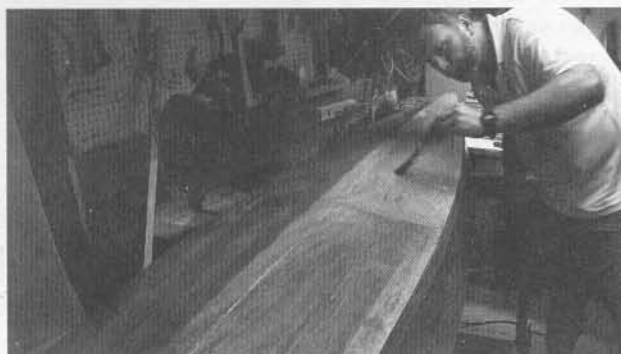
Saturate the hull with epoxy resin, using a foam roller, then tip out any runs and bubbles with a disposable bristle brush.
