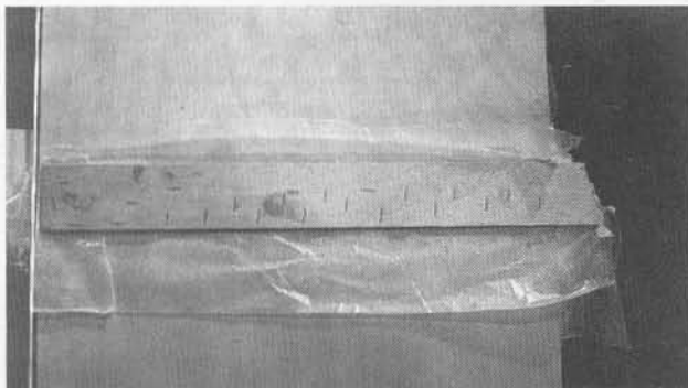
Clamping the scarf by stapling it to the work surface is quick and easy. The piece of scrap plywood will be pulled up with all the staples once the epoxy has cured. Notice the string line used to check alignment.
