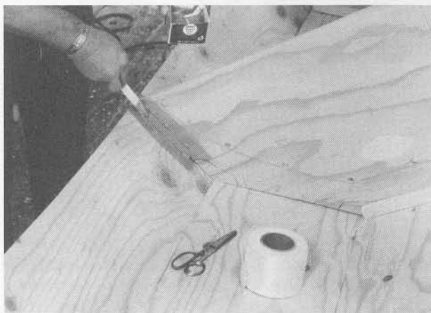
With the top cleat removed, use putty to create a fillet between the frame and the side panel.
