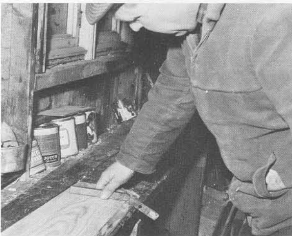
The planed plank is checked with a sliding bevel set to the appropriate mark on the bevel board.
