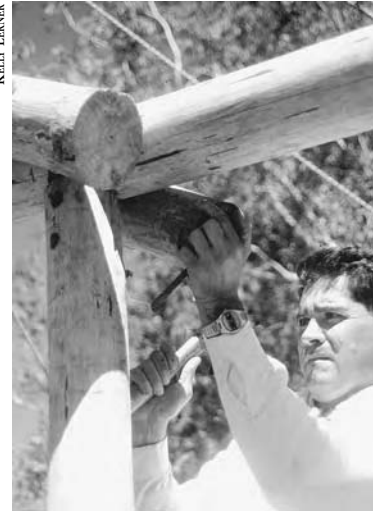
7-20: Small-diameter wood poles create the structure for a straw bale house in Argentina.
