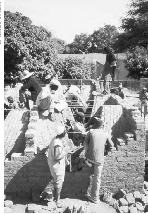
5-2: Development Workshop uses special training structures to educate students about the basics of woodless construction. In this example in Mali, students learn how to build vaulted roofs of adobe bricks.
