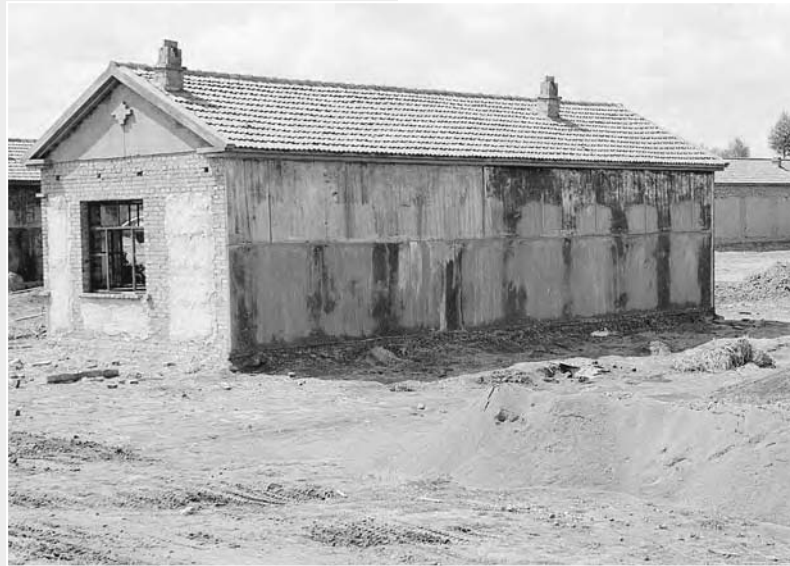
5-16: Lime plaster drying on a brick and bale house. Note the differential drying rates.
