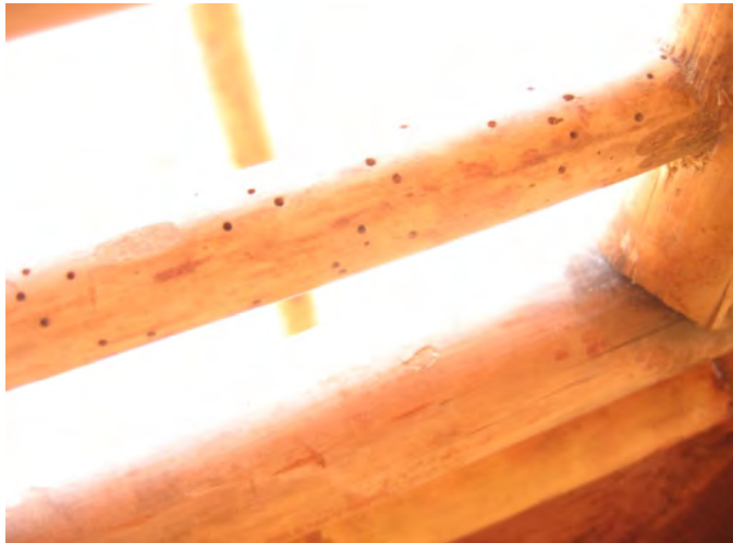
Figure 31 - Borer beetle exit holes
