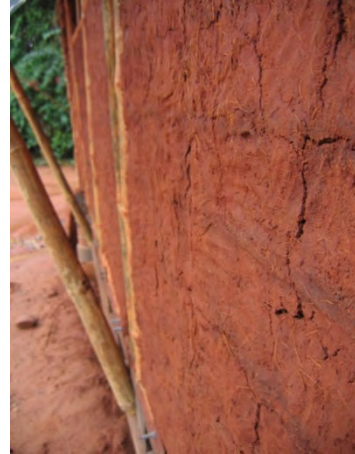
Figure 22 - Cracks appeared and could be filled
