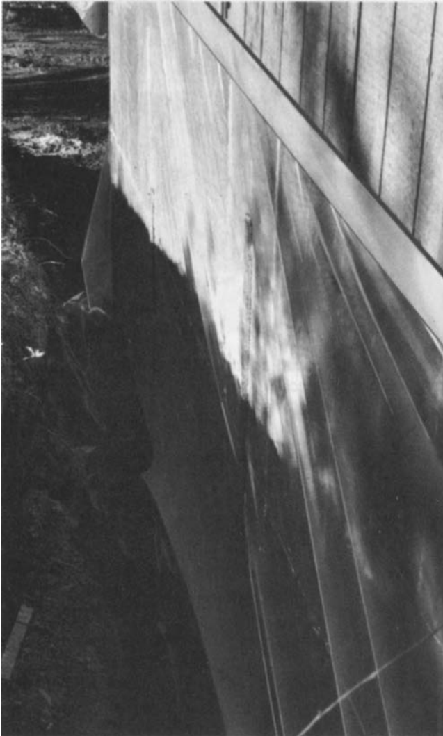
Figure 3-25 Polyethylene secured to exterior of PWF with 12-inch pressure treated grade strip. (Courtesy Wood Products Promotion Council)
