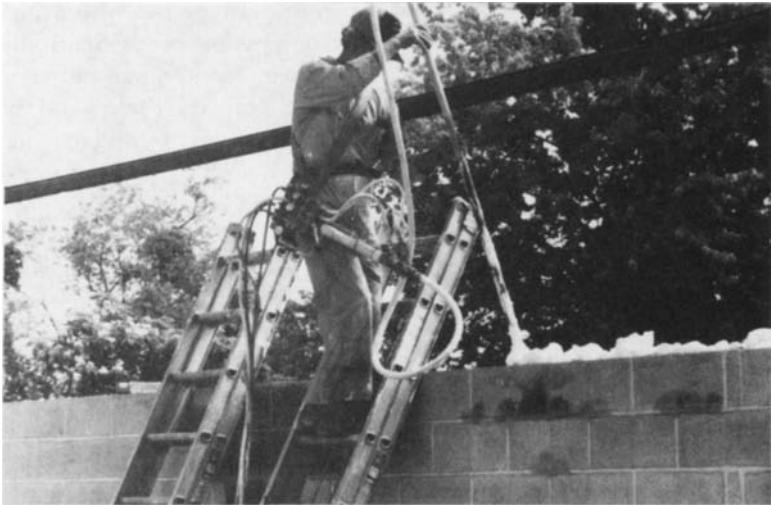
Figure 17-15 Air Krete cement-based insulating foam being installed in concrete blocks. (Courtesy Palmer Industries, Inc.)
