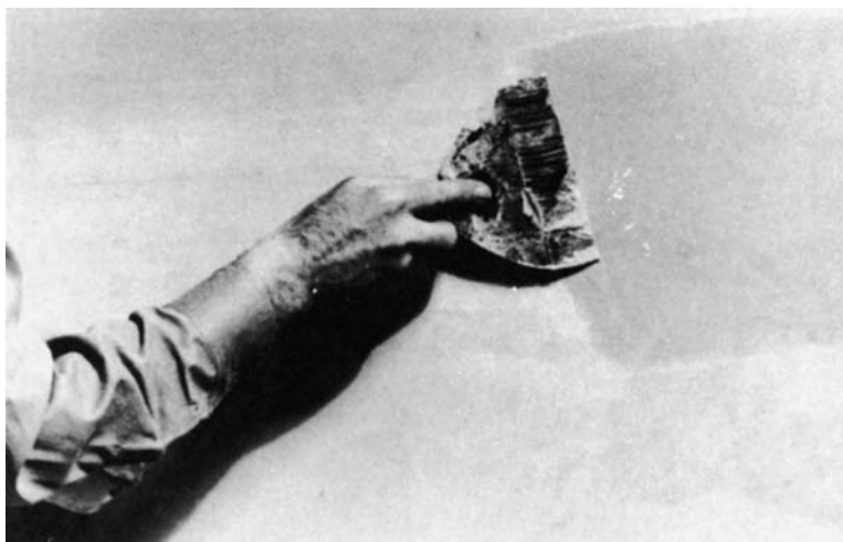
Figure 18-30 The final coat is applied with a wide knife, carefully feathering edges. A wet sponge will eliminate need for further smoothing when dry. (Courtesy National Gypsum Co.)
