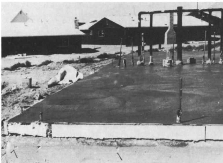
Figure 4-9 Finished slab of a home under construction. Water and sewer pipes were placed before concrete was poured.
