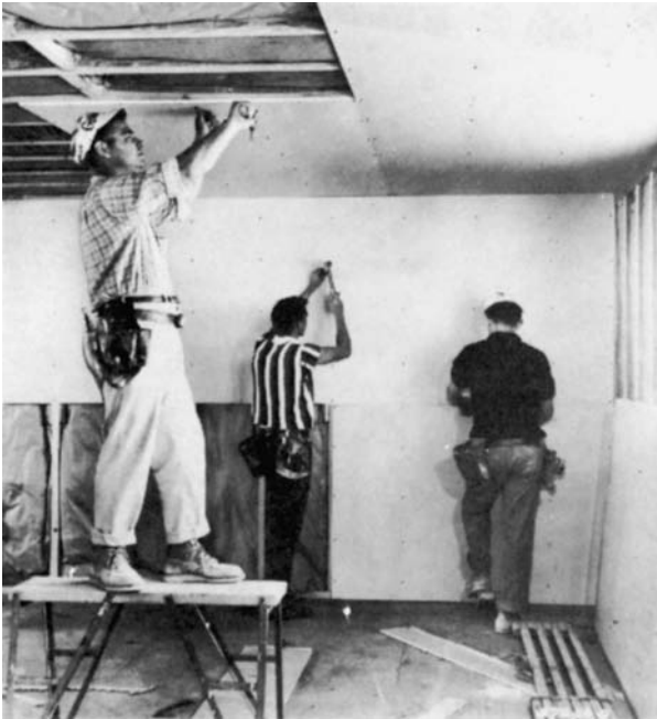
Figure 18-2 The most common interior finishing uses plasterboard, known as drywall construction. (Courtesy National Gypsum Co.)
