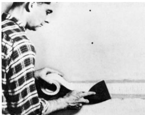
Figure 18-26 Place perforated tape over the joint and embed it in the joint compound. (Courtesy National Gypsum Co.)
