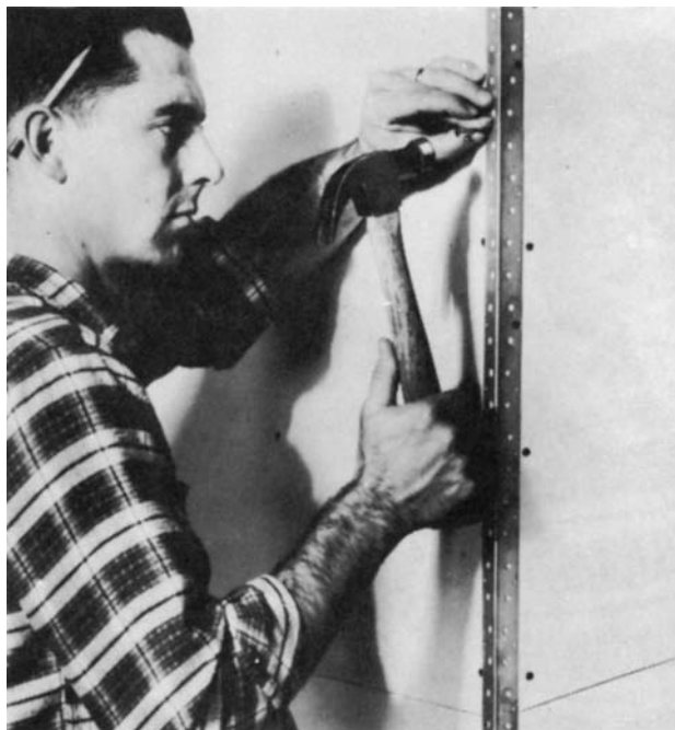
Figure 18-32 Outside corners are generally reinforced with a metal bead. It is nailed in place through the plasterboard into the stud. (Courtesy National Gypsum Co.)
