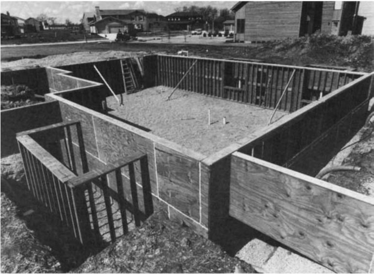
Figure 3-26 A completed PWF ready for concrete slab and floor platform, before backfilling. (Courtesy Wood Products Promotion Council)
