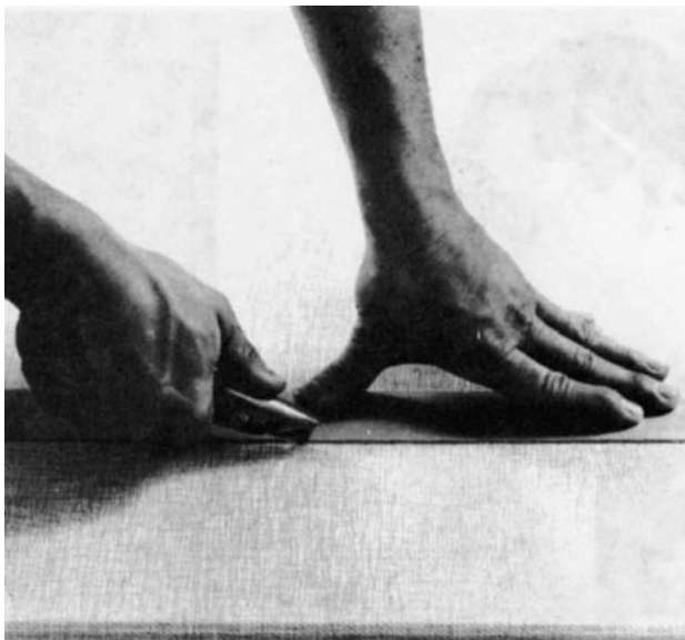
Figure 18-34 When cutting vinyl-finished wallboard, the cut should be about 1 inch wider than the desired width. This is to allow an inch of extra vinyl for edge treatment. (Courtesy National Gypsum Co.)
