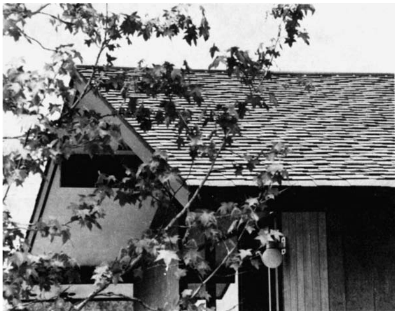
Figure 13-3 These asphalt shingles have a three-dimensional look. Asphalt shingles are the most popular.
