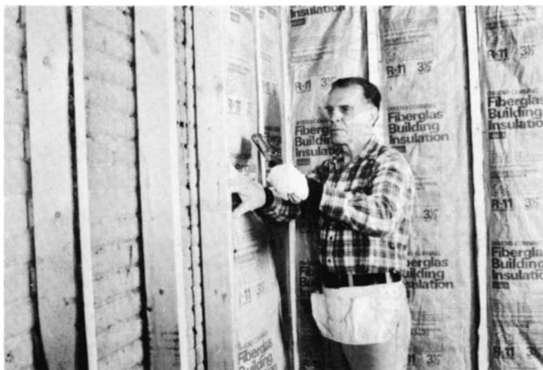
Figure 17-12 Properly installed insulation.
