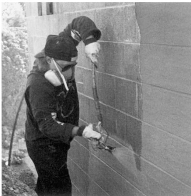
Figure 3-12 Spraying the Rub-R-Wall onto the outside of a concrete block basement wall.
