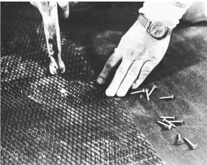
Figure 22-11 In this installation, mesh is secured to floor. Cement is to be used. It is an old-fashioned mud job.
