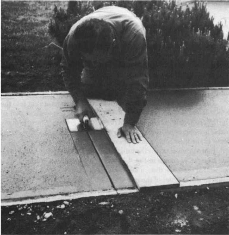
Figure 4-6 Cutting a groove in a walk. If any cracking occurs, it will be in the groove, where it is less conspicuous.
