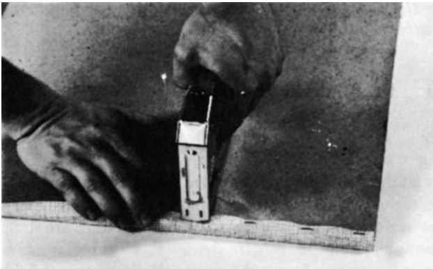
Figure 18-36 Fold the 1-inch vinyl material over the edge of the wallboard and tack in place. This will provide a finished edge without further joint treatment. (Courtesy National Gypsum Co.)
