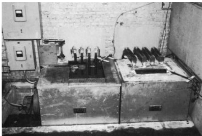
Figure 10-10 Typical installation of two electrode-type pot furnaces.
