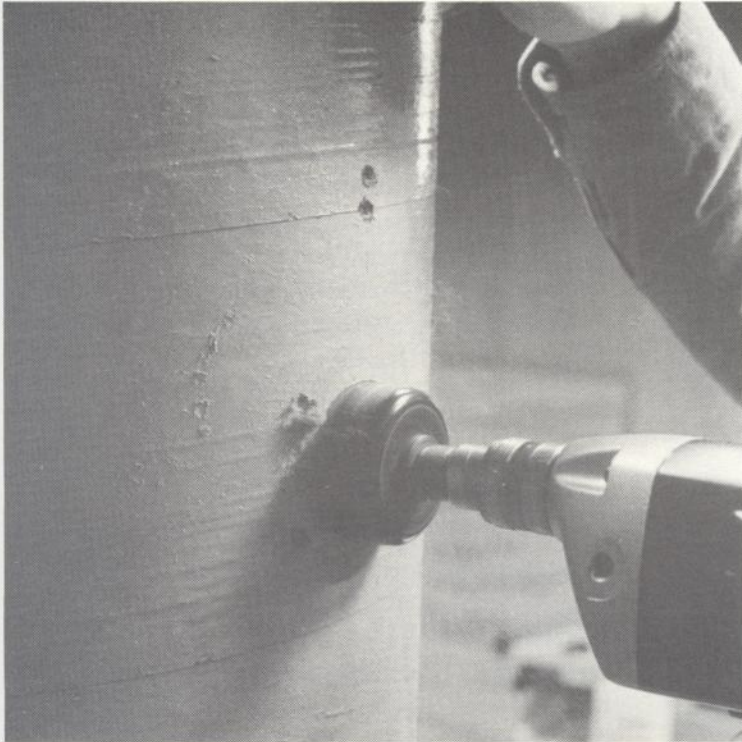
Before applying the second coat of paint, drill all openings in the tube.
