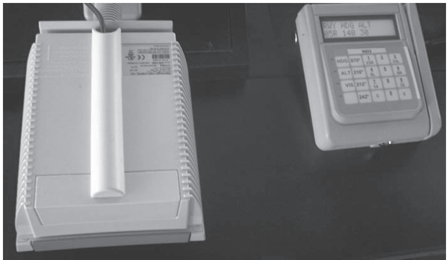
Figure 10–12. Bar code reader in control tower.
