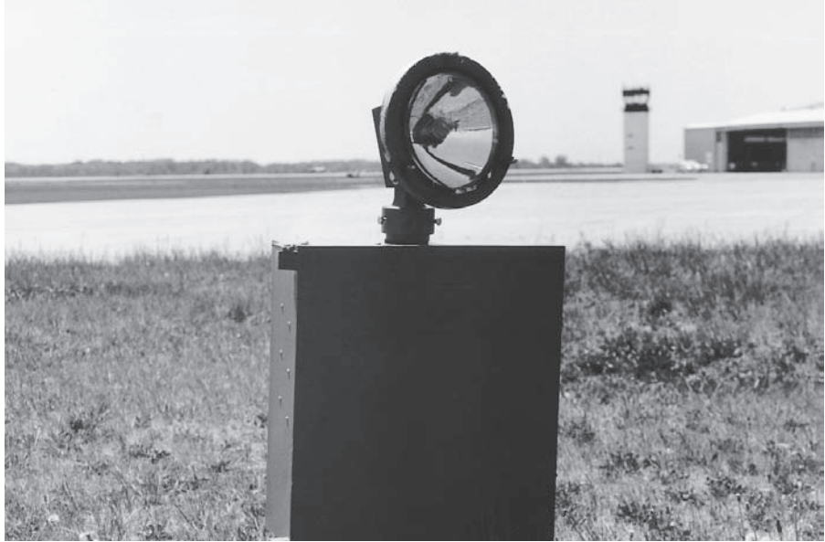
Figure 2–74. A typical runway end identifier light installation.
